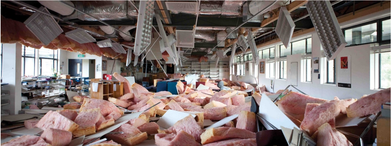
Figure 1: Non-structural damage following the Mw 6.1 2011 Christchurch earthquake
