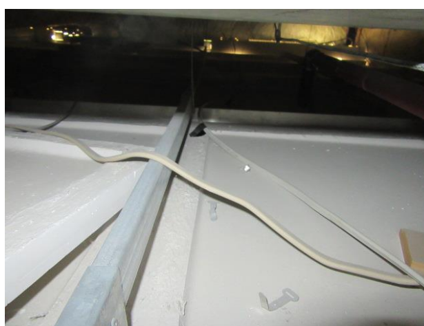
Electrical wires laid directly on ceiling.
