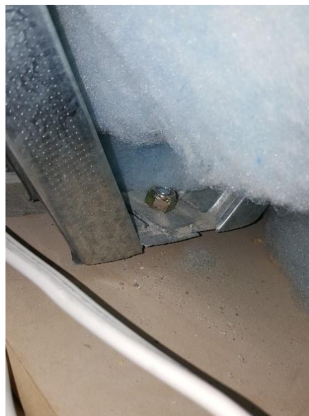
Partition bracing, no clearance around penetration suspect fasten
