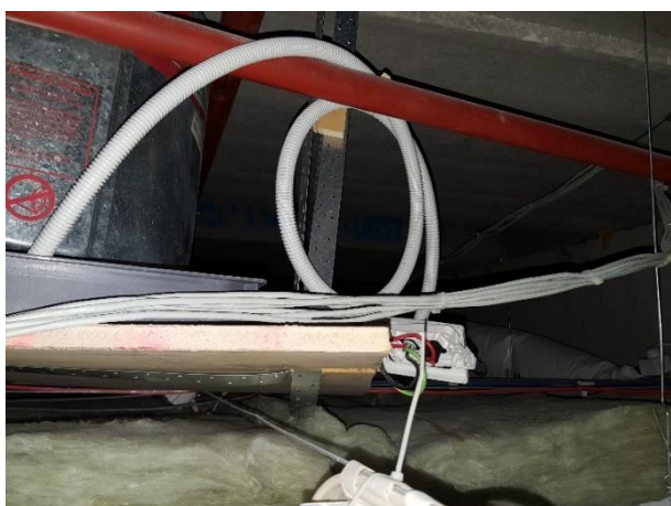
Water tank on a swing could interact with sprinkler
