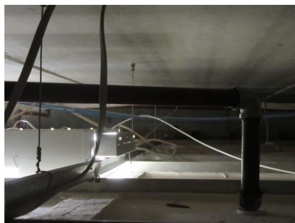
Fire Range End not supported independently; supported by ceiling only. Light fitting not supported or restrained independently.
