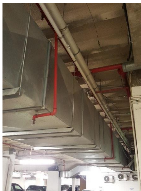
Interaction between ducting and fire sprinklers likely.
