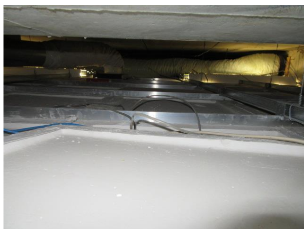
No ceiling bracing present. Cables leading down into unrestrained partition wall and unrestrained soft ducting in background.
