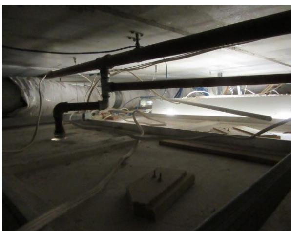
Fire sprinkler within 150mm of slab, unrestrained light (not supported independently), soft ducting unrestrained over 3m length.
