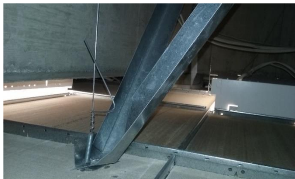
Partition wall poorly braced
