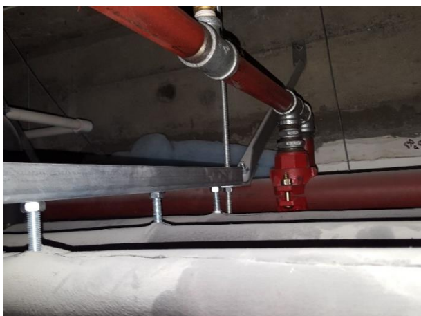
Pipework trapeze; inadequate clearance to fire
