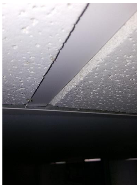
Grid ceiling to rondo ceiling not fastened
