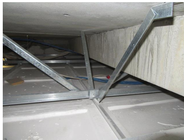
Ceiling bracing. Weakest element is 3.6mm aluminium rivet fastening to grid. Dynabolts in Hollowcore also failing
