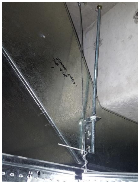
Large ducting could interact with ceiling hangers
