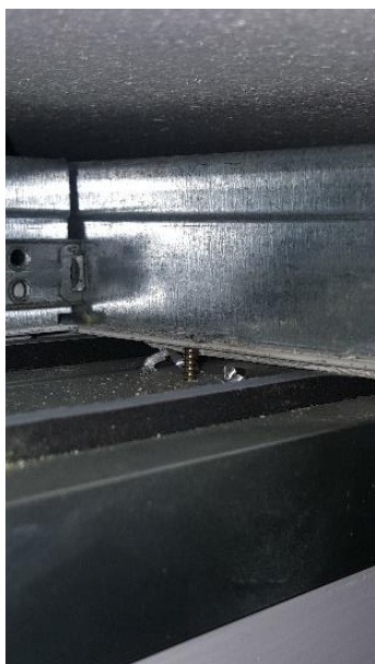
Typical wall to ceiling fasten. This appears to have sheared.
