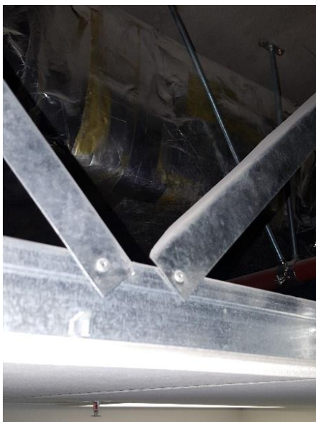
Ceiling bracing let down by weak fastener at element, note poor angle of fire brace in back ground
