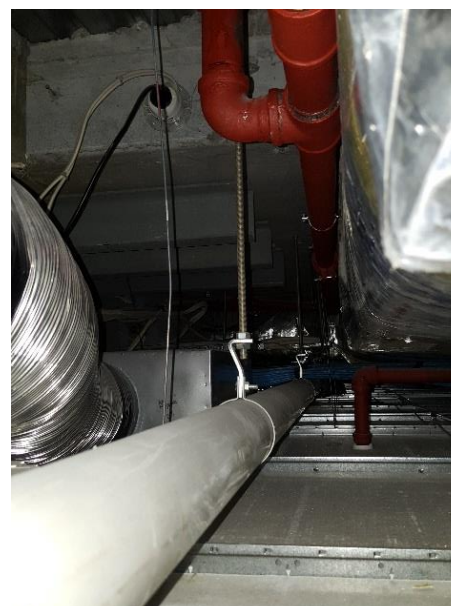
Ceiling bracing let down by weak fastener at element, note poor angle of fire brace in back ground
