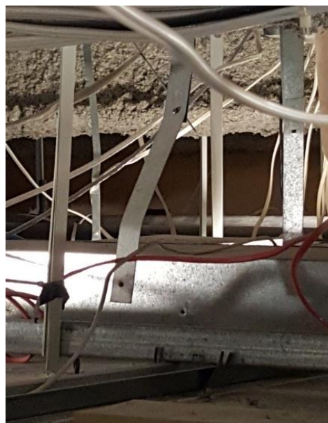
Duct hanger rivet fail
