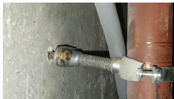
Failing in hollowcore, previous drift evident
