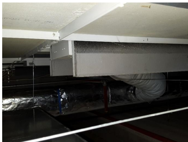
Large lighting not independently supported
