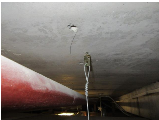
6mm Dynabolt pulling out of Hollowcore concrete slab
