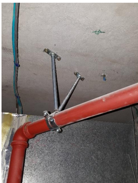
Ceiling bracing let down by weak fastener at element, note poor angle of fire brace in back ground
