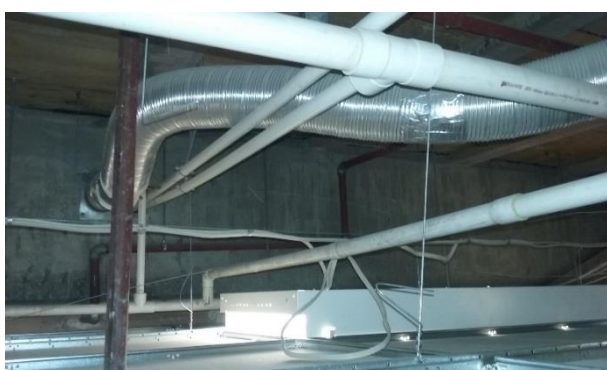
Range ends not braced, Light not braced Pipe work not braced or supported.
