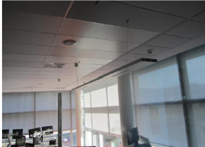
Figure 9: Typical suspended luminaire
