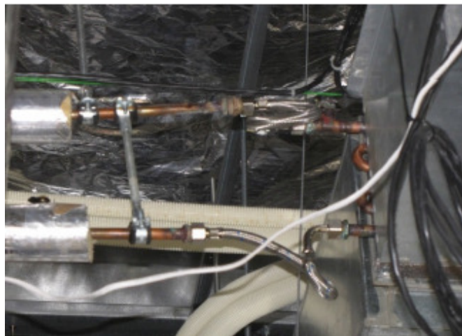
Figure 6: Use of flexible connections on mechanical plant to achieve compliant installation
