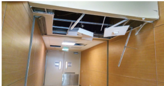
Figure 13: Ceiling damage in hospital corridor link
