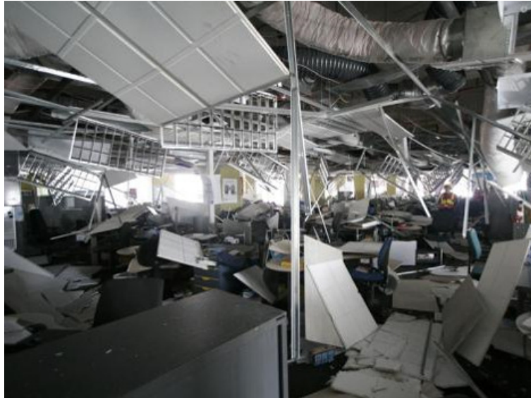
Figure 4: Failure of ceilings and services in Christchurch commercial building
