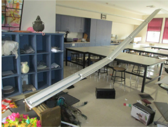
Figure 15: Damaged light fixtures - commonly observed in school facilities
