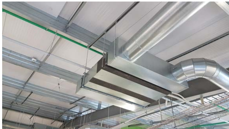
Figure 16: Non-compliant installation of overhead mechanical plant (no lateral restraint provided) – building completed and received Code Compliance Certificate 2015
