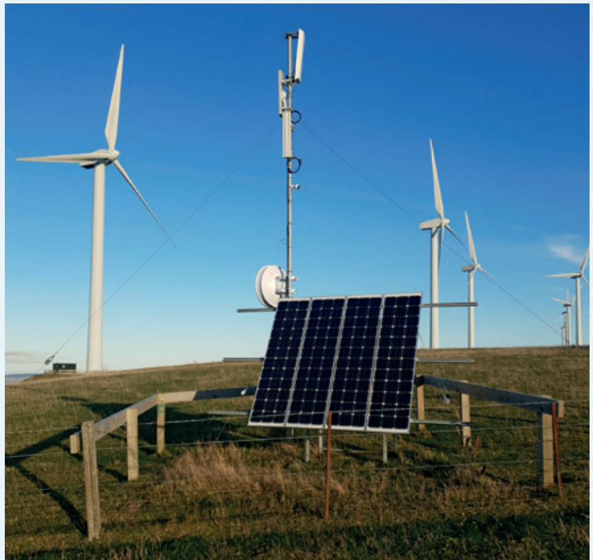
This antenna on Mt Stewart shares its windy location with nine wind turbines.
