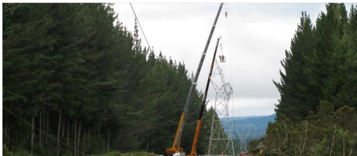
Figure 4: Damage to Bunnythorpe-Wairakei 'A' line near Rangipo in 2012
