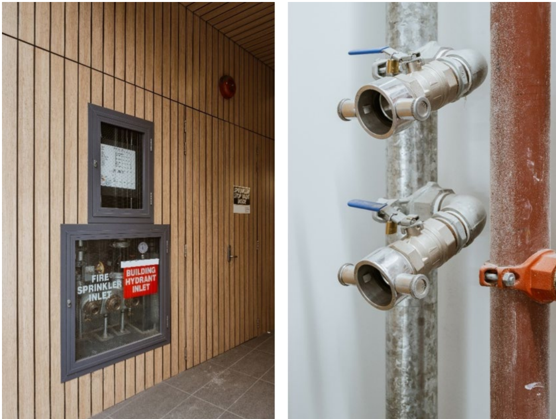
Figure 18. Fire alarm panel, sprinklers and hydrant inlets, and internal hydrants
