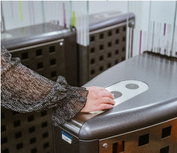
Figure 16. Speed gate access controls requiring a card
