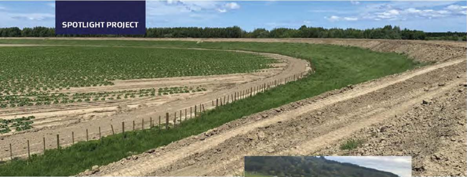
Construction of a section of the Waipaoa stopbank, protecting a large area of crops.
