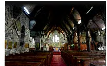
Figure 2. View of the Cathedral nave showing internal face stone walls and timber roof structure
