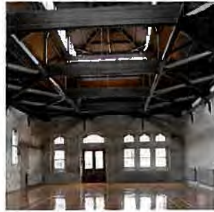
Figure 6. Steel bracing at eave level used to strengthen the Christchurch Arts Centre gymnasium
