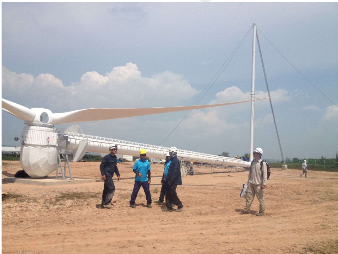
Figure 7.3. Photo of the tilt-up XANT turbine.
