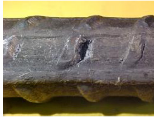
Figure 12: Surface cracks and deep cracks
