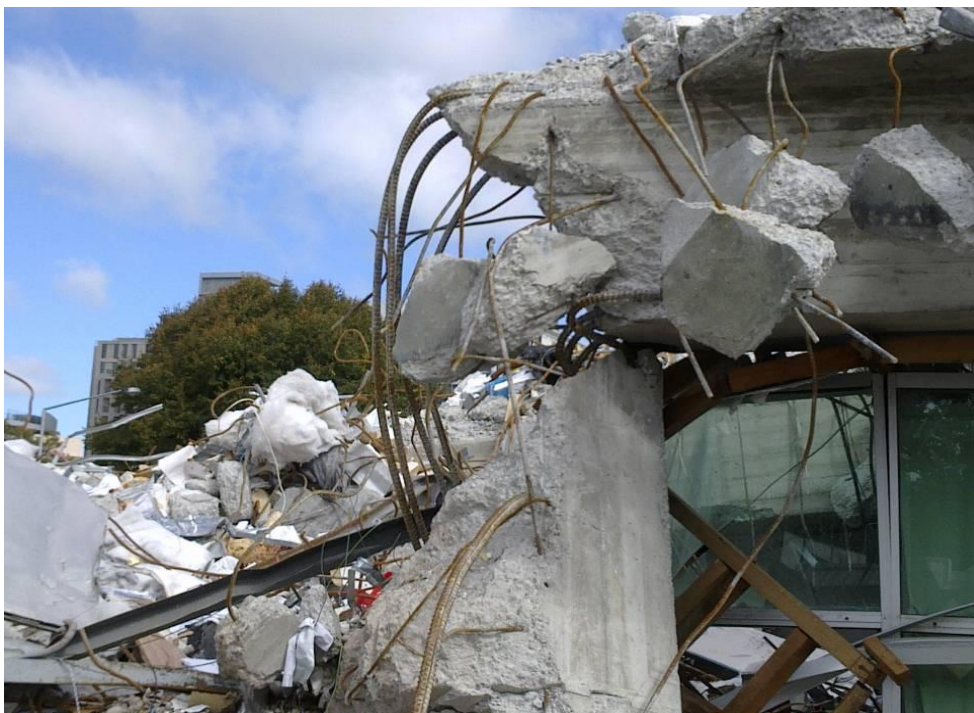
Figure 12 - Sheared concrete beam attached to portion of floor still standing
