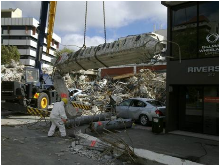
Figure 1 – Structural concrete beam remnant being moved by mobile crane and site crew wearing personal protection equipment due to presence of asbestos.
