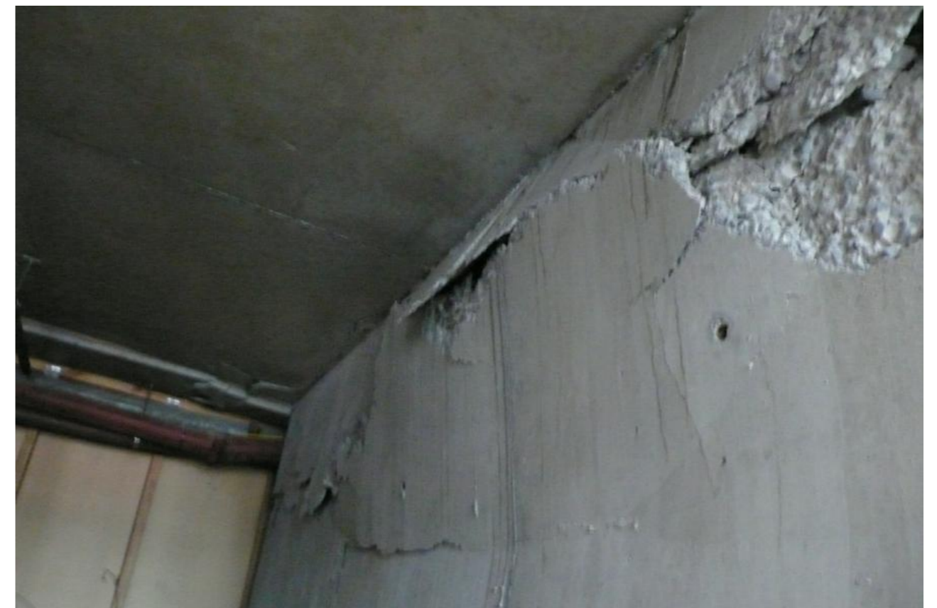
Photo 8 - Shearwall D5-6 - Hingeing at top of ground floor
