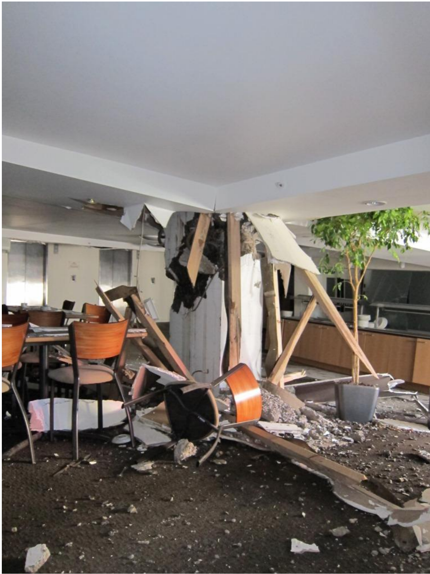
Photo 20 - Crushed columns at level 10, lines 5 & 6
