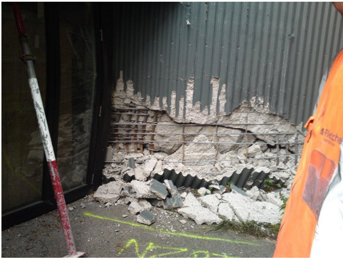
Photo 11 - Similar Shearwall Failure Not the Hotel Grand Chancellor
