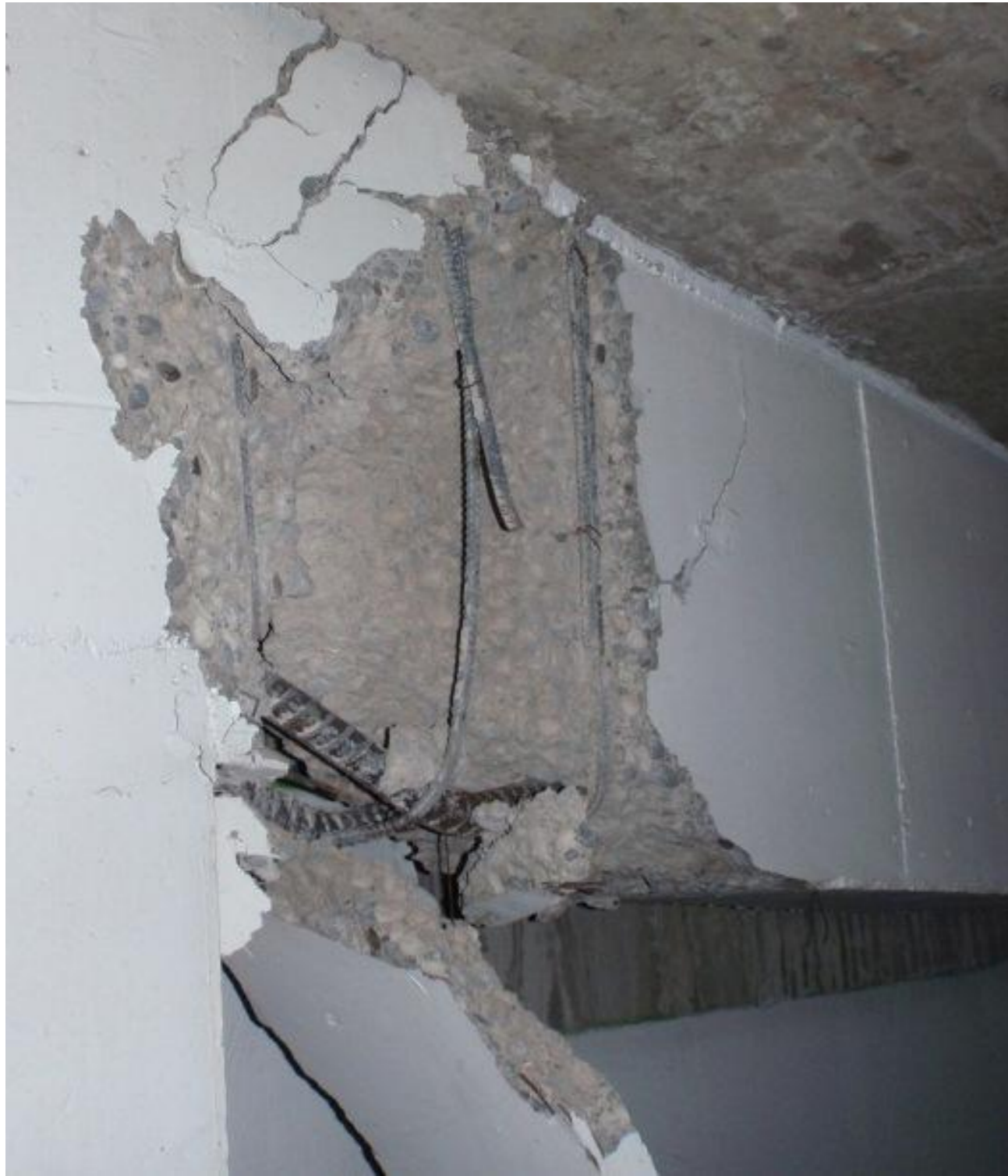
Photo 14 - Hingeing in grid E beams 6-7
