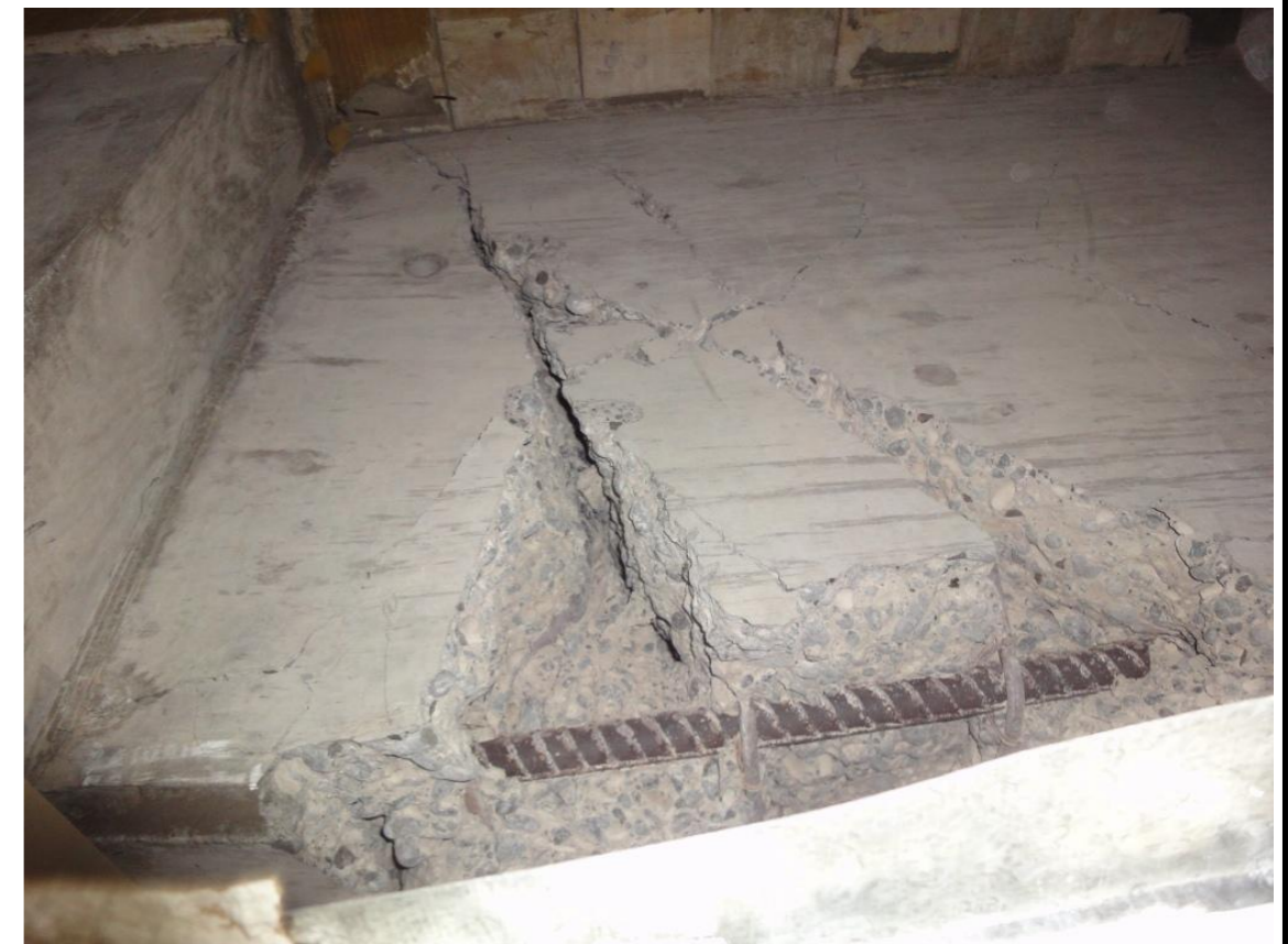
Photo 19 - Hingeing in grid D tower beams
