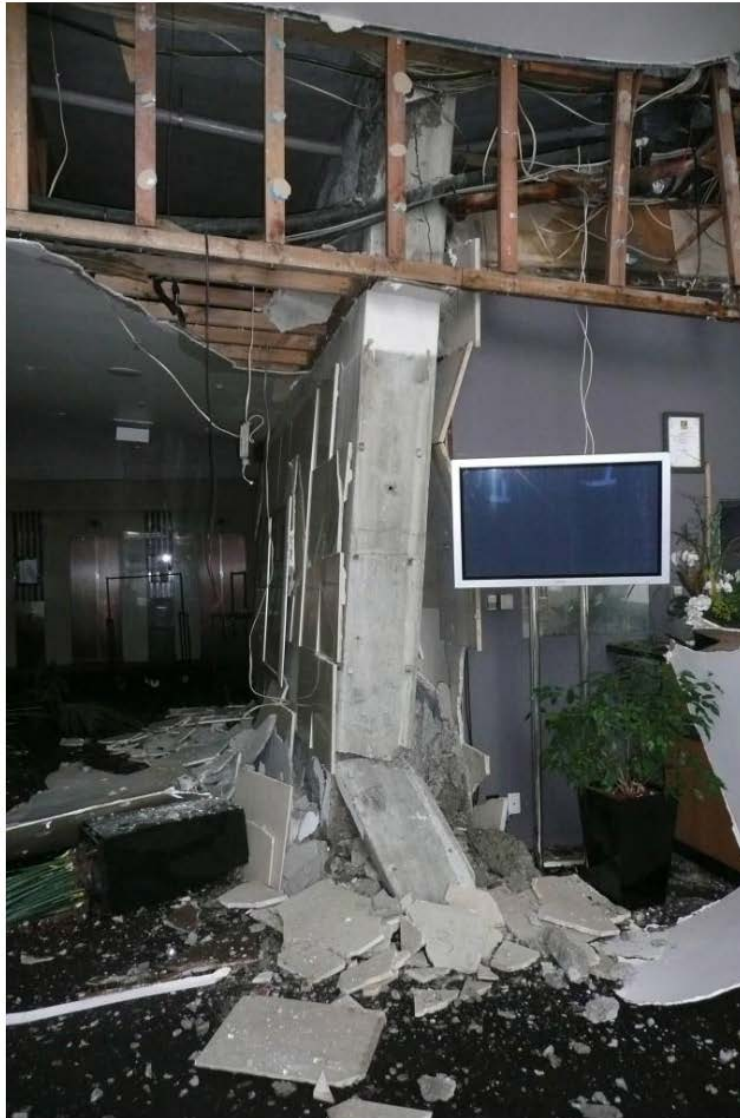
Photo 6 - Shearwall D5-6 - Base Failure
