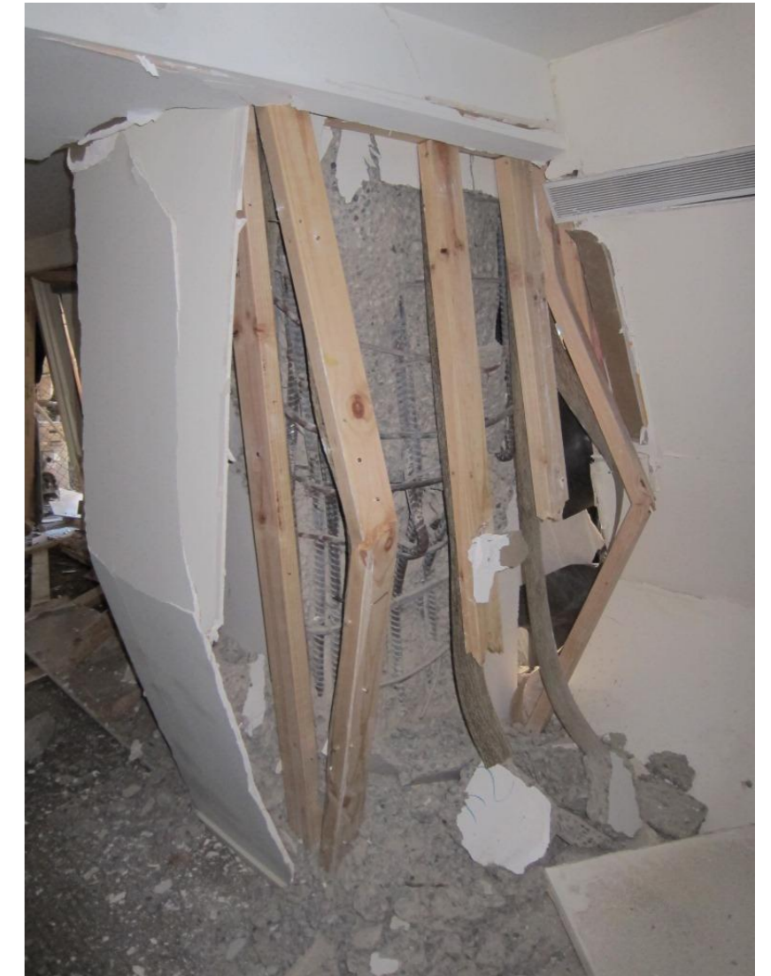
Photo 21 - Crushed columns at level 10, lines 5 & 6
