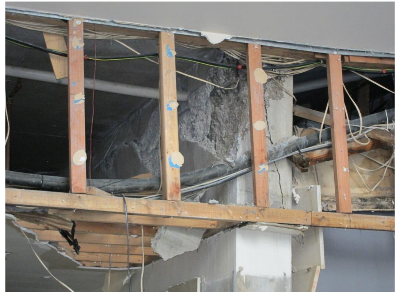
Photo 7 - Shearwall D5-6 - Hingeing at top of ground floor
