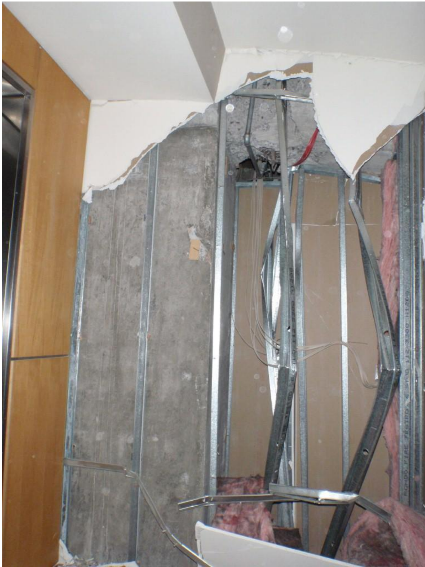
Photo 17 - Hingeing in grid D tower beams
