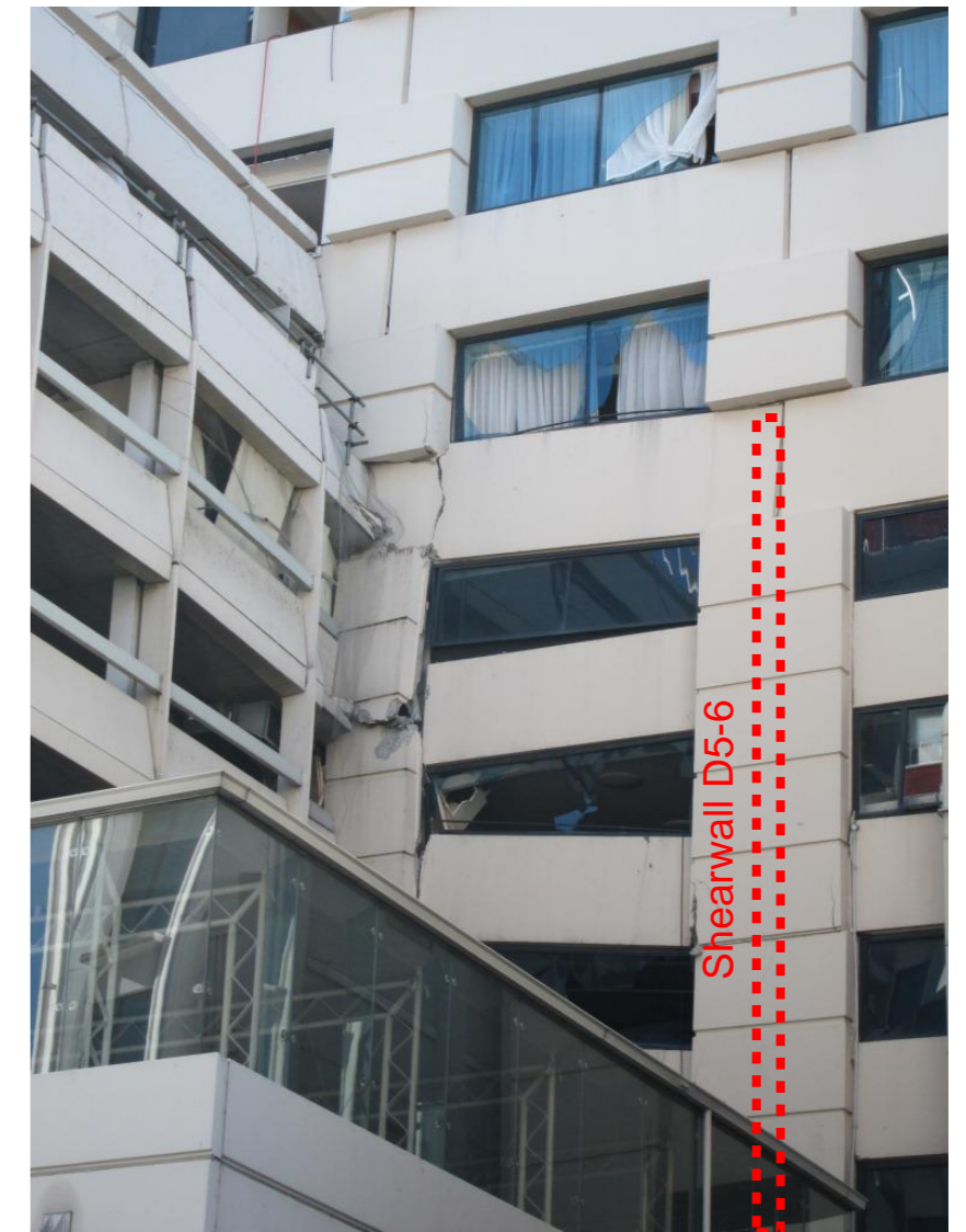
Photo 5 - Damage at junction between podium and tower - not related to pounding
