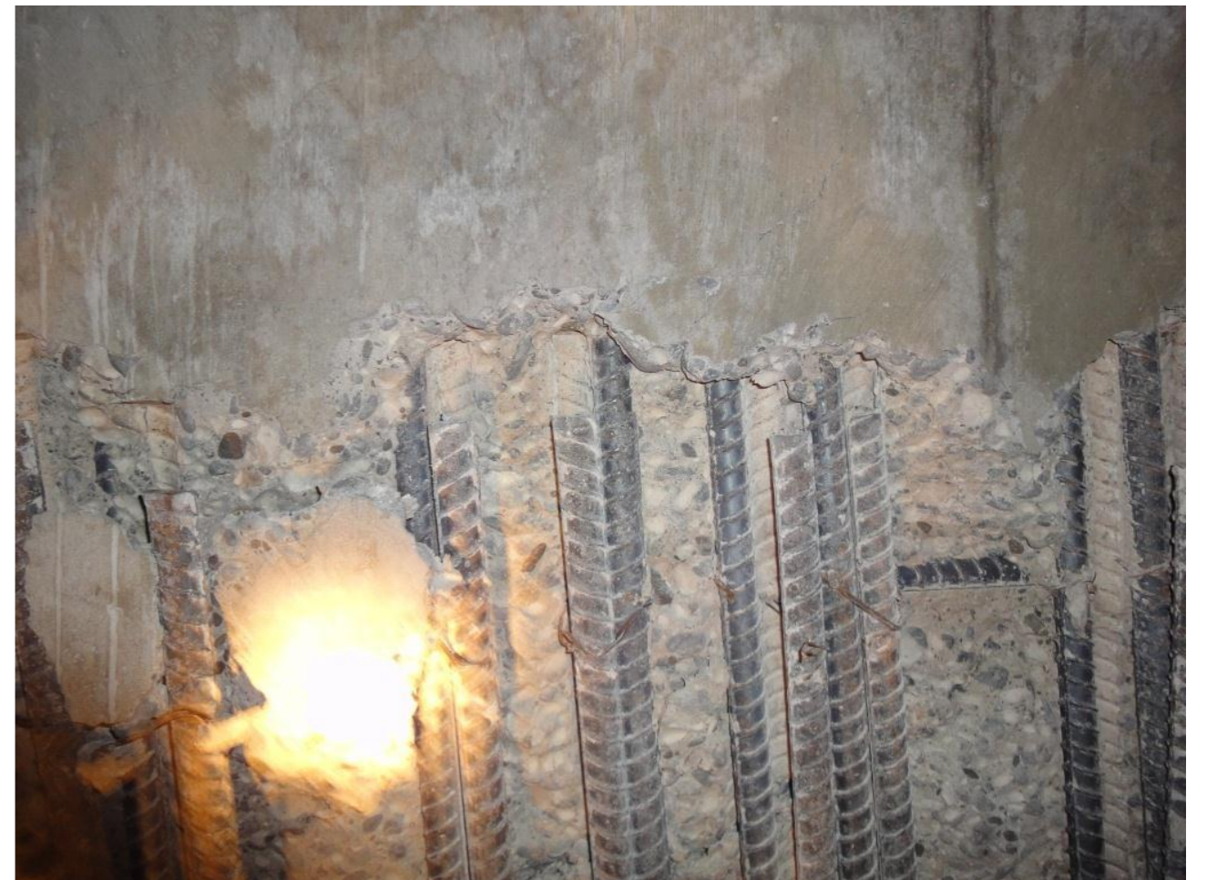
Photo 16 - Near-lap failure grid 8 cantilever transfer beam
