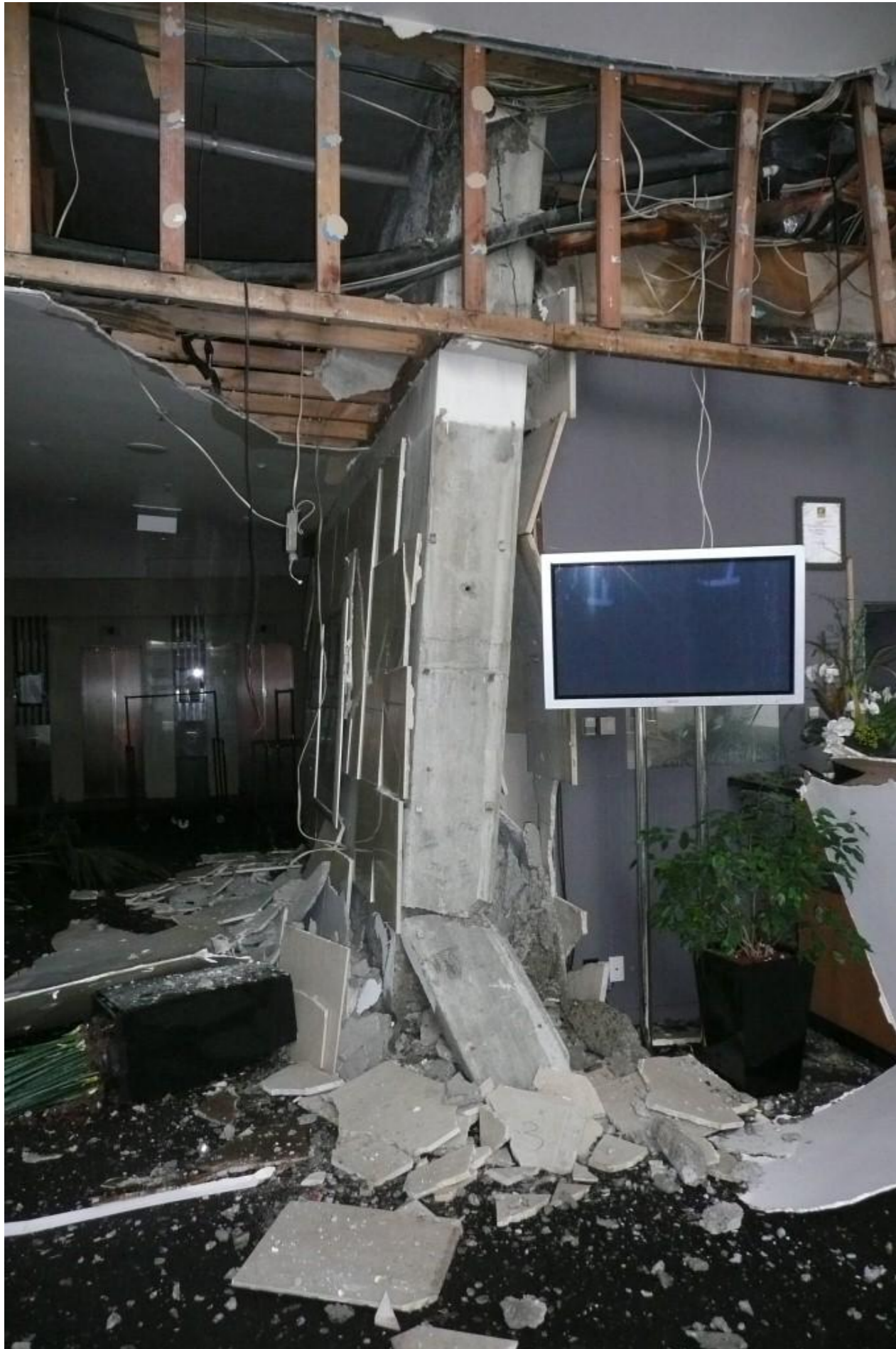
Photo 6 - Shearwall D5-6 - Base Failure
