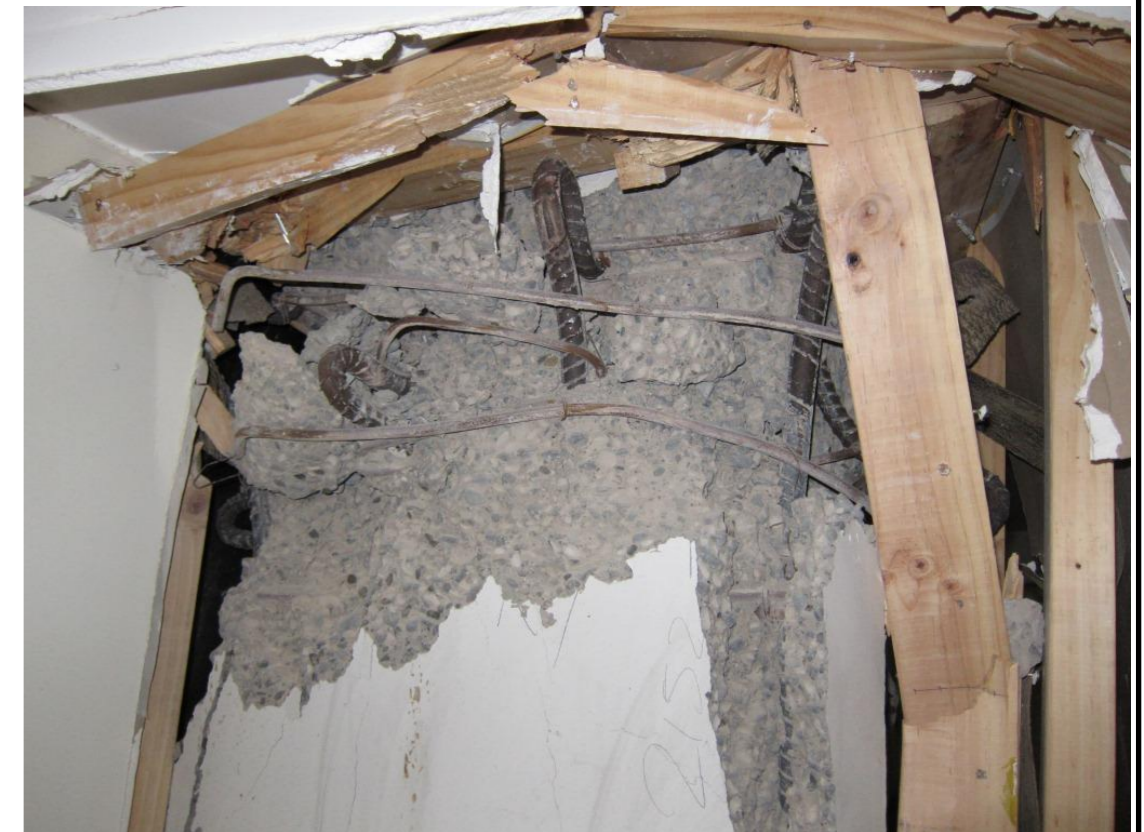
Photo 22 - Crushed columns at level 10, lines 5 & 6
