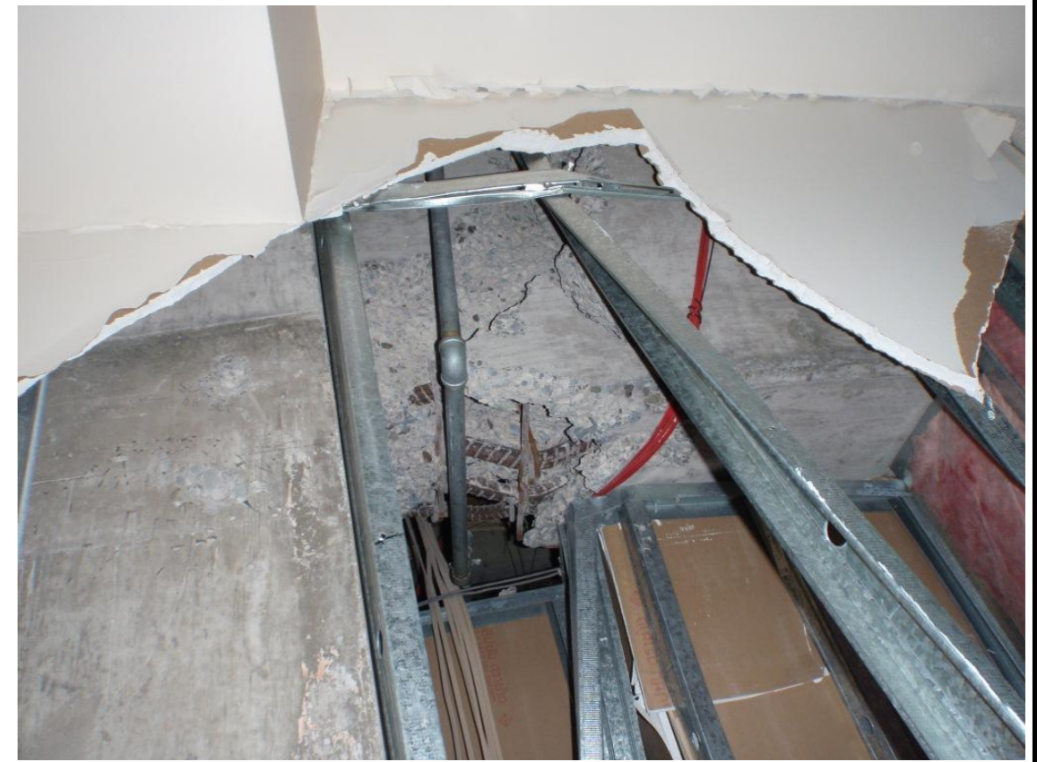
Photo 18 - Hingeing in grid D tower beams
