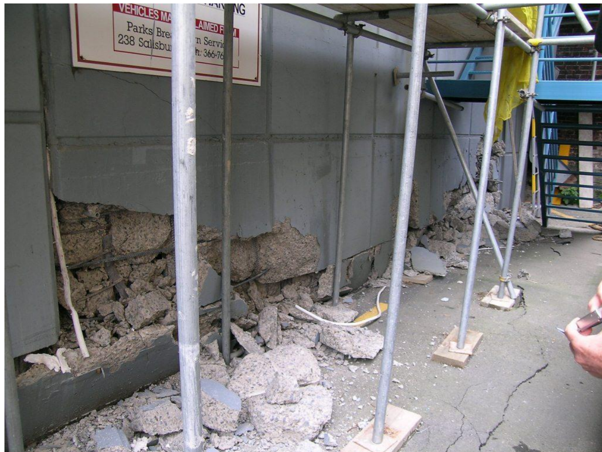
Photo 12 - Similar Shearwall Failure Not the Hotel Grand Chancellor
