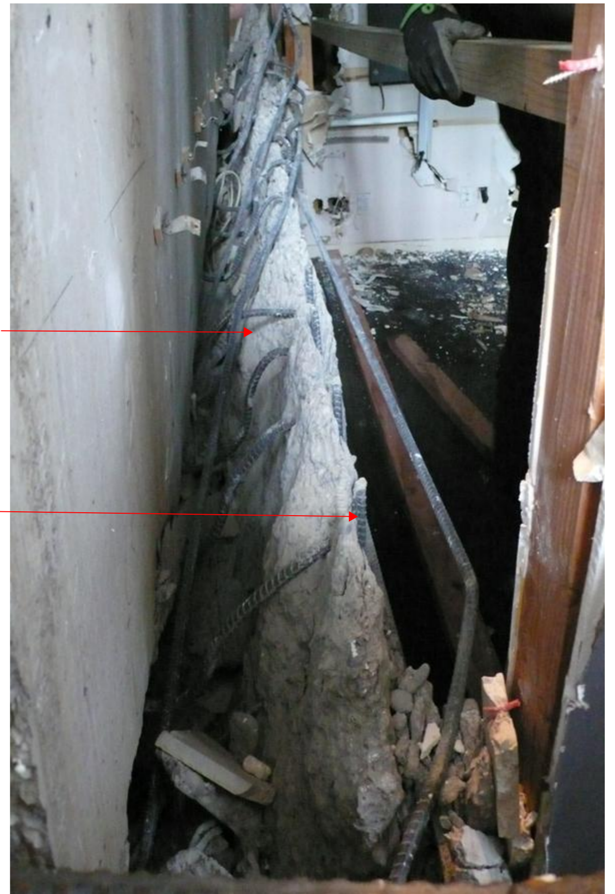
Photo 10 - Shearwall D5-6 Failure - Close-up
