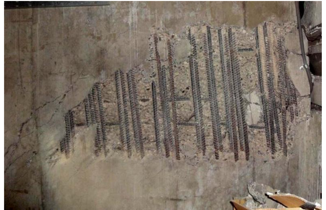
Photo 15 - Near-lap failure grid 8 cantilever transfer beam
