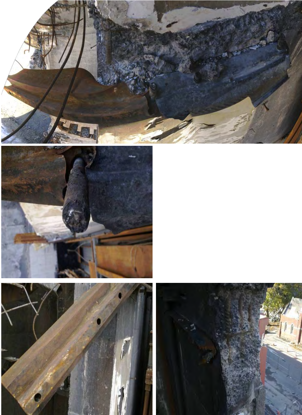
Figure 39 - Level 5 Lift Well Wing Walls Grid D and D/E (anti-clockwise from top) (a) 150x150x10 L with 51 x 3.2 SHS; 4-M24 bolts into wall and 6 –M20 threaded rods 350 mm long fixed through the slab at the profiled metal deck rib with epoxy grout around rod; Three M20 threaded rods remained vertical the Grid D Drag Bar. The 51x3.2 SHS had fractured in bending and tension at the bolt hole adjacent to last bolt into wall and twisted with the slab; (b) Epoxy grout around threaded rod in slab; (c) Holes for 3-M20 threaded rods in slab in twisted Drag Bar; d) 150x75x10 L Drag Bar with 5-M24 threaded rods fixed into wall D/E. End of Drag Bar had been gas cut during deconstruction.
