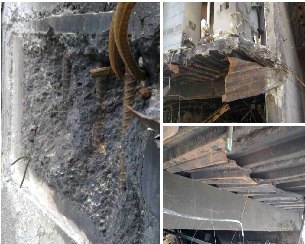
Figure 29 - Line 4 North Core Walls Level 4 slab remnants (top to bottom) (a) Connection of shell beam to wall with two fractured H24 top bars and two de-bonded top bars. No bottom bars from shell beam embedded in wall but imprints from bars evident (DENG B23 Dwg S18 (Figure 67), Detail 5 S19 (Figure 71)), corresponding to the bent back bottom steel in shell beam Item E23 (Figure 8); (b) Fractured vertical face of slab at stairwell wall, with fractured slab support beam (DENG B25 Dwg S18 (Figure 67)) top bar and charred fracture surface; (c) Torn profiled metal deck sheeting de-bonded from slab but still fixed in at pre-cast beam support.
