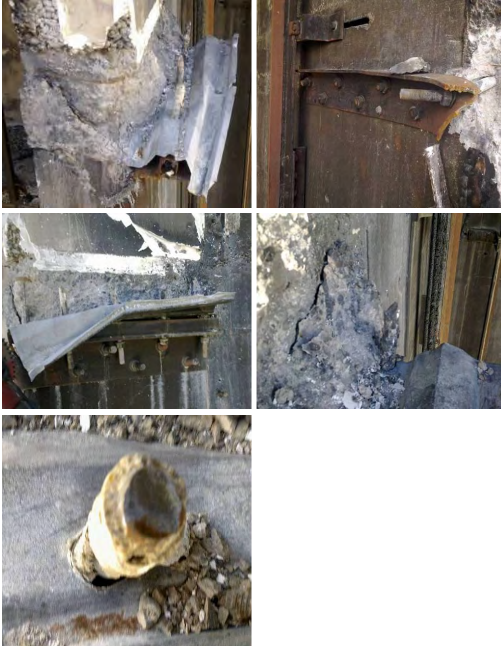
Figure 40 - Level 6 Lift Well Wing Walls Grid D and D/E (anti-clockwise from top left) (a) 150x150x10 L with 51 x 3.2 SHS into west wall on Grid D, similar to Level 5 and 4 Drag Bars; 6-M24 bolts into wall; The remaining 4 -M20 bolts 350 mm long had been fixed into the slab at the profiled metal deck rib with epoxy grout around bolt; These remained vertical and were measured with 110 mm stick-out above the item. The 51 x3.2 SHS has fractured in bending and tension at the bolt hole adjacent to last bolt into wall and the bar had twisted with the slab; (b) Side view of Drag Bar remnant showing deck uplift at end bolt; (c) Top surface of M20 threaded rod with typical smooth diagonal face and grout around rod through slab. (d) End rod with diagonal top surface and slab concrete remains; (e) 150x75x10 L Drag Bar with 7- M24 threaded rods fixed into east wall D/E. End of bar had been gas cut during de-construction.
