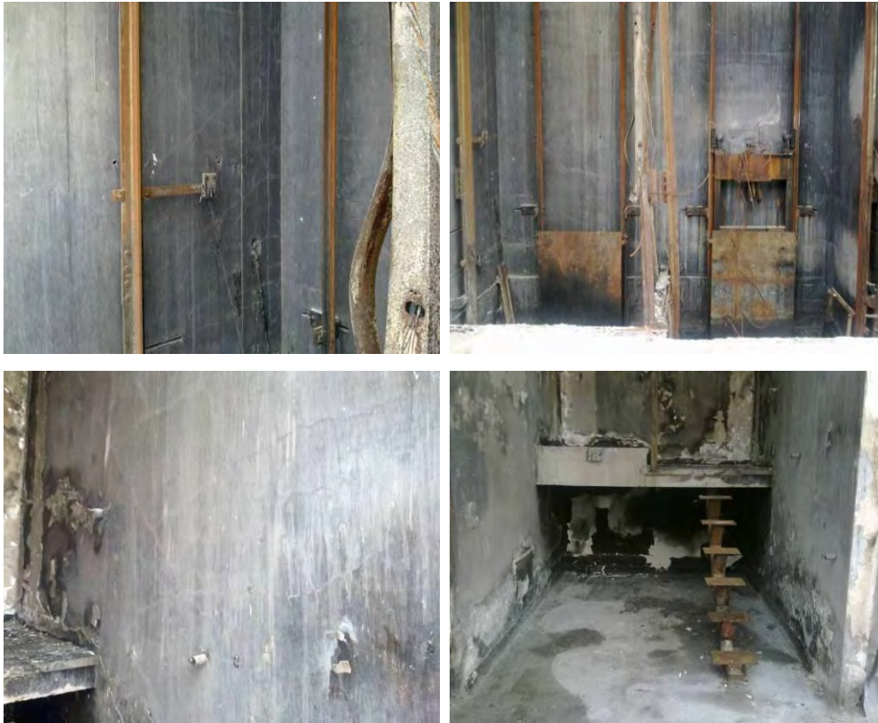
Figure 26 - Lift and Stair well wall cracking Level 1 to Level 2 (clockwise from top left) (a) Lift wall face of Line D wall with fine diagonal shear cracking in both directions; (b) Lift wall face of Line 5 wall with fine diagonal cracking in both directions; (c) Stairwell area with steel stair stringer where concrete cores were extracted; (d) Stair well face of Line D wall with fine diagonal cracking in both directions.
