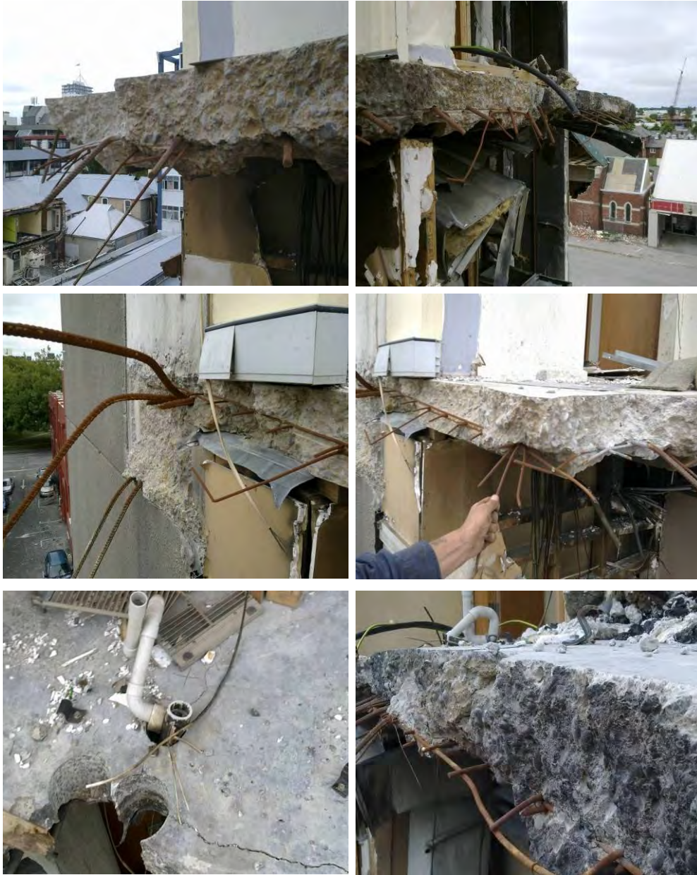
Figure 28 - Line 4 North Core Wall Slab Remnants Level 5 (clockwise from top left) (a) West end with H12 bar ends and mesh at bottom of slab above ribs. It was required on the drawings to be located near the top surface (DENG Dwg S16 (Figure 75)); (b) Looking east. Reinforcing angled down; (c) Slab edge on Grid C west end. Mesh angled down in bottom of slab on top of ribs; (d) Fire charred vertical fractured slab edges adjacent to stairwell. Mesh located low down in slab at top of slab ribs. Edge of mesh sheet with closely spaced parallel wires exposed. Fractured wires can be seen from the lapped mesh below; (e) Cracking in slab running from cored holes; (f) Connection of shell beam to wall with two fractured H24 top bars and two de-bonded top bars. No bottom bars from shell beam embedded in wall (DENG B23 Dwg S18 (Figure 67), Detail 5 S19 (Figure 71)), corresponding to the bent back bottom steel in shell beam Item E23 (Figure 8).
