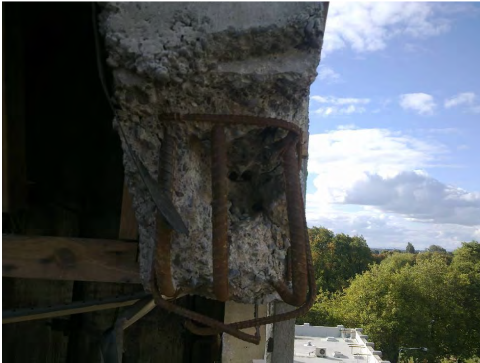
Figure 41 - Lift Well Wing Wall D/E: Column D/E 4 Connection (DENG Dwg S14 (Figure 69); 3 x 20 to 24 mm diameter holes could be seen where reinforcing bars from the column had pulled out. The drawing shows that 4-H20 bars were required to be bent into the wall.
