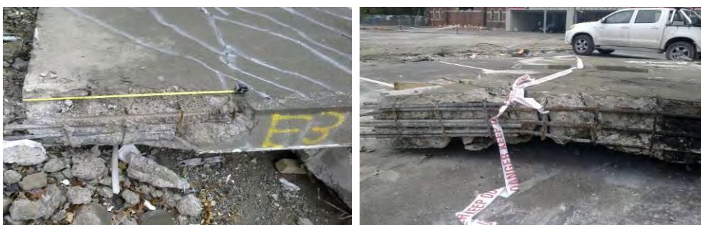
Figure 44 - Locations of H24 reinforcing bar samples (left to right) (a) East end of Line I South Wall item E3, one cut from lower 1050 mm of wall; (b) Two lapping bars from lower E3 wall item taken from east end of wall item E4
