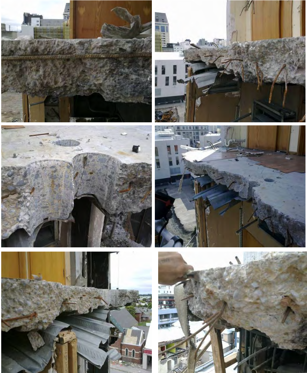
Figure 27 - Line 4 Core Wall Slab Remnant at Level 6 amenity area (clockwise from top left) (a) Slab edge on stairwell wall looking west with H12 saddle bar exposed and ends of mesh below it; (b) Vertical concrete fracture surface with reinforcing mesh fractured; (c) Slab looking west with cores cut in floor for amenities; (d) Fractured mesh angled downwards; (e) Fractured slab edge looking east. Torn metal decking aligned approximately with concrete fracture edge; mesh at varying height within slab; (f) Cores for amenities at fracture edge.
