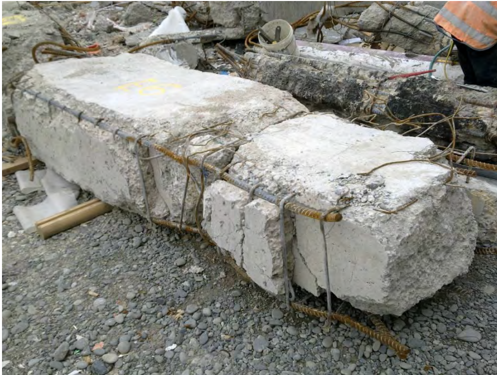
Figure 6 - Edge shell beam Item E6 showing unreinforced concrete infill and smooth interface between shell beam and in-fill. The DENG Specification Precast Concrete cl 3.12 required roughened interface surfaces (Figure 77).
