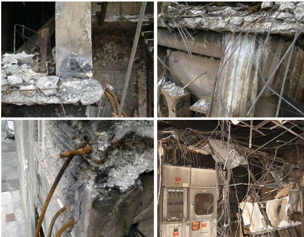
Figure 31 - Line 4 North Core Walls Level 2 slab remnants (clockwise from top left) (a) Slab edge broken back during de-construction adjacent to stairwell wall; (b) Broken back slab with H12 saddle bars exposed. Masonry wall with separation along top course; (c) Switch room under Level 2 slab; (d) Connection of shell beam to wall with two fractured H24 top bars and one de-bonded top bars. Bottom bars from shell beam have been embedded in wall as specified (DENG B23 Dwg S18 (Figure 67), Detail 5 S19 (Figure 71)). Some diagonal beam-wall joint zone shear cracking can be seen in the wall end..
