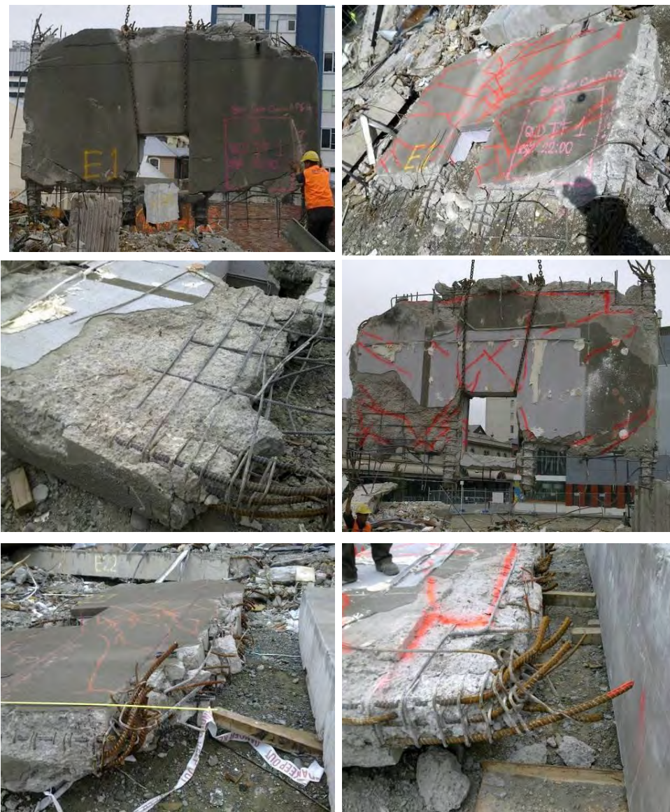
Figure 14 - Line Shear Wall (Item E1) (clockwise from top left) (a) Outer face of wall with lower portion of concrete removed during deconstruction exposing the reinforcing steel; (b) Outer face with cracks highlighted by red paint; (c) Inside face with cracks highlighted by red paint; (d) Top west corner; (e) Top east corner; (f) Inside face of east pier
