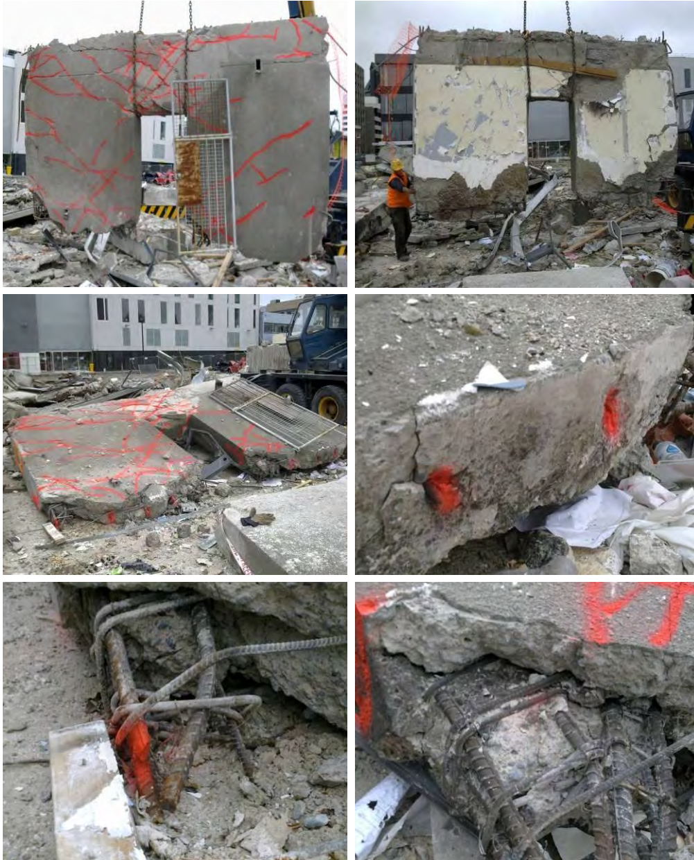
Figure 16 - Line 1 South Wall Level 2 to Level 3 (Item E2) (clockwise from top left) (a) Outside face with fire escape door attached. Cracks marked by red paint; (b) Inside face of wall; (c) East pier construction joint with necked and fractured bars indicated by red paint; (d) Escape door edge of east pier showing thick cover concrete to reinforcing; (e) Outer edge of west pier showing necked and fractured bar indicated by red paint others were cut; (f) Outer face of wall with cracks and fractured bars marked.
