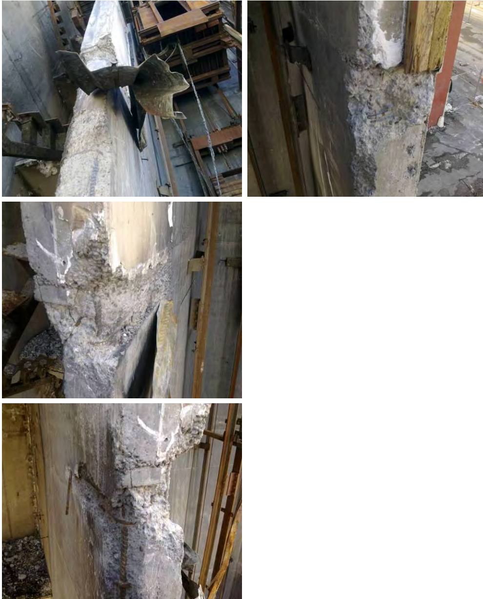
Figure 35 - Level 3 Lift Well Wing Walls Grid D and D/E (anti-clockwise from top left) (a) Profiled metal deck decking side lapped into western Grid D wall, just hanging on; (b) H12 bar necked and fractured at centre of wing wall (indicated by chalk arrow); (c) Concrete cover appeared to have broken away as the slab pulled southwards; (d) Localised spalling of concrete. No reinforcing found connecting end of east wall with slab.
