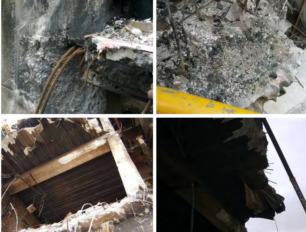
Figure 30 - Line 4 North Core Walls Level 3 slab remnants (clockwise from top left) (a) Connection of shell beam to wall with two fractured H24 top bars and two de-bonded top bars. No bottom bars from shell beam embedded in wall but imprints from bars evident (DENG B23 Dwg S18 (Figure 67), Detail 5 S19 (Figure 71)), corresponding to the bent back bottom steel in shell beam Item E23 (Figure 8); (b) Ash on slab; Cored holes at fractured edge; (c) Torn profiled metal deck sheeting de-bonded from slab but still fixed in at pre-cast beam support (DENG B24 Dwg S18 (Figure 67)); (d) Profiled metal deck and slab from below supported on beam B24.
