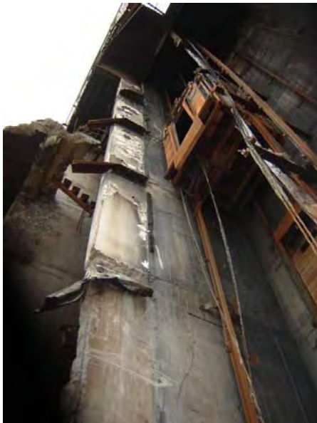
Figure 33 - Drag Bar connections at Levels 6, 5 and 4 on lift well west wing wall on Grid D. No Drag Bar at Level 3 or 2 (Figure 32)
