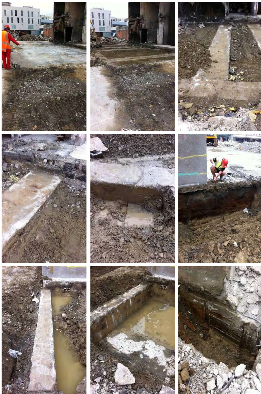
Figure 60 - Foundation Inspection (From left to right in rows from top) (a) P947; (b) P948; (c) P968; (d) P971; (e) P960; (f) P903; (g) P964; (h) P919; (i) P993
