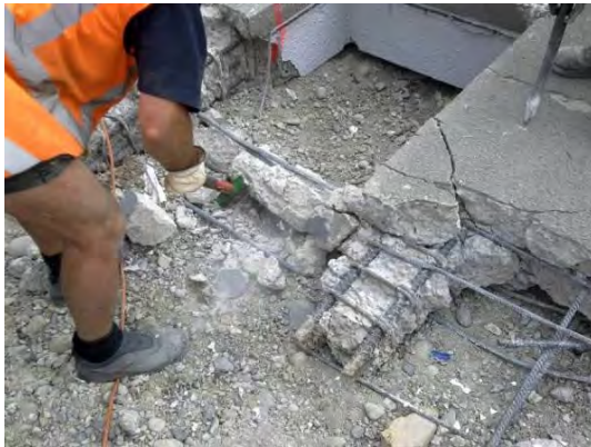
Figure 42 - Line 1 South Wall Item E1 H16 bars from masonry door infill.
