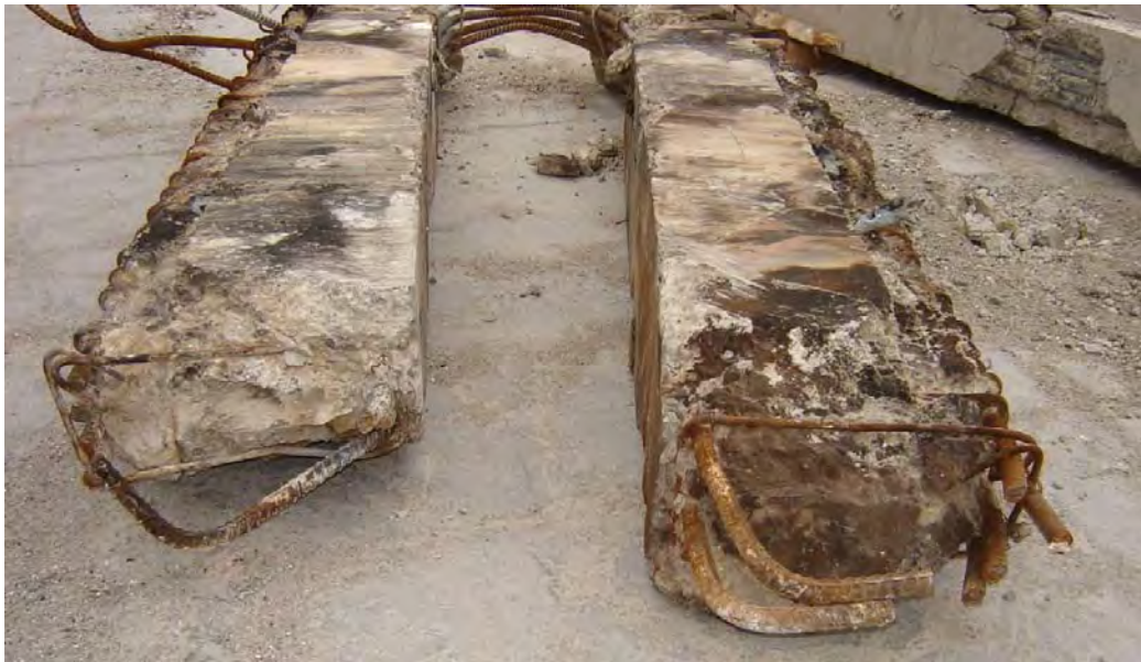
Figure 12 - Interior Pre-cast Log Beams from Line 2 and 3 (DENG Section 3 Dwg S15 (Figure 66)) showing smooth concrete formed for beam-column joint and bottom hooked bars that have pulled out of beam-column joints without any obvious straightening; metal decking has pulled away from slab seating; no slab remains attached to the beams
