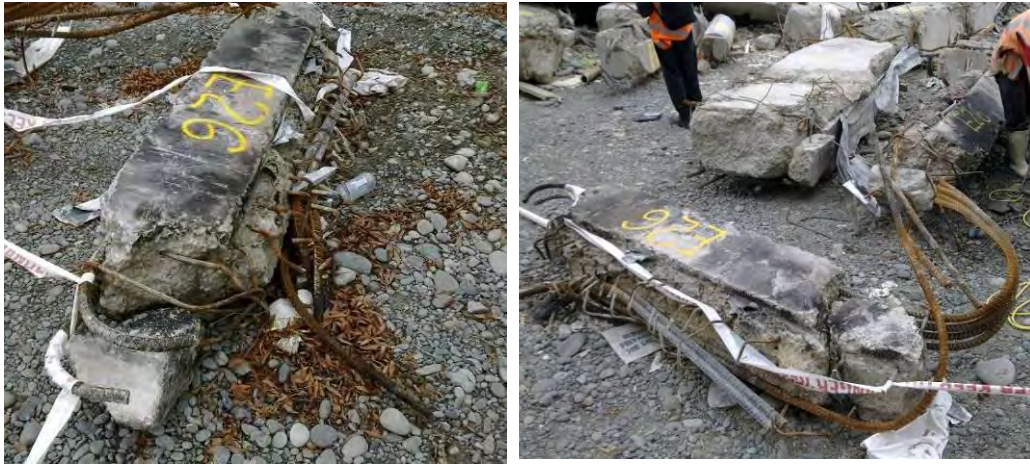
Figure 11 - Interior Pre-cast Log Beam from Line 2 and 3 (DENG Section 3 Dwg S15 (Figure 66)) (left to right) (a) Diagonal shear damage at end and smooth formed surface at beam-column joint; (b) Mid-portion of beam concrete has broken away and stirrups are pulled apart.
