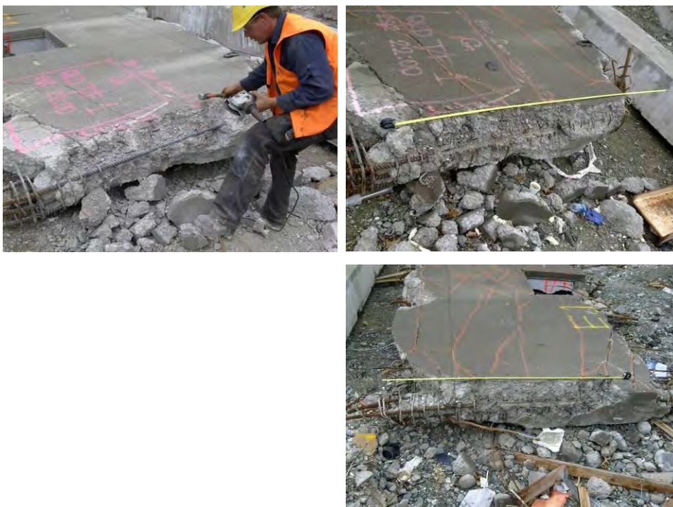
Figure 43 - H28 from east and west end of Line I South Wall Item E1 (clockwise from top left) (a) H28 about to be cut from east end (EIE); (b) Top of 1000 mm long EIE sample 1300 mm from top of L2 slab; (c) Top of 1000 mm long EIW sample from west end 750 mm from top of L2 slab. Coupling beam depth was 1700 mm.
