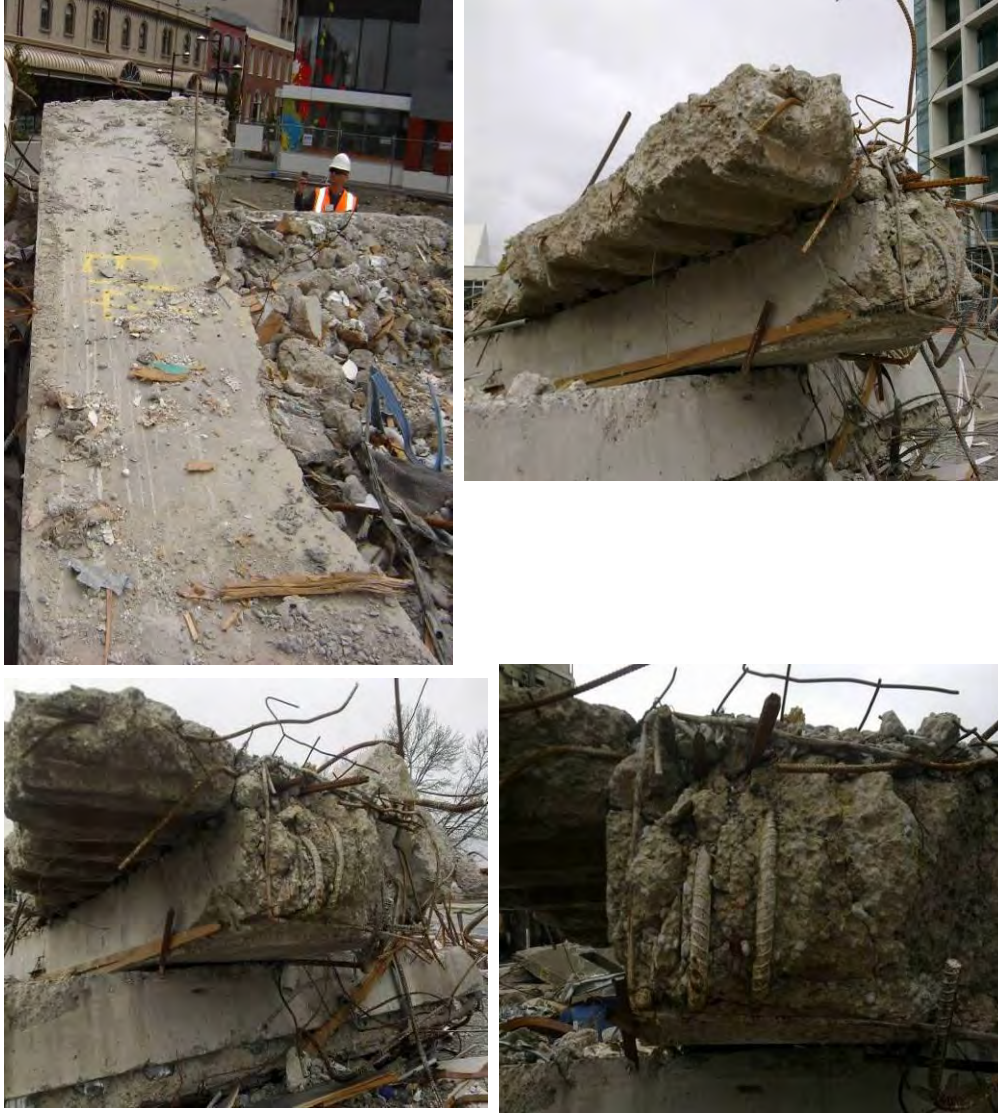
Figure 7 - Pre-cast shell beam (Item E14) from northern face Grid 4, west side of lift core (DENG B23 Dwg S18 (Figure 67)). (clockwise from top left) (a) Top face with slab fracture along edge of shell beam, extending out further at far end adjacent to lift core attachment; (b) to (d) Fractured slab outstand remnant at east end from which slab concrete cores were extracted. The bottom H24 bars from shell beam have been turned back into the concrete infill rather than embedded in shear wall as specified (DENG Detail 5 Dwg S19). Refer also bar imprint on wall at the connection seen in Figure 29 at Level 4 and Figure 30 at Level 3.
