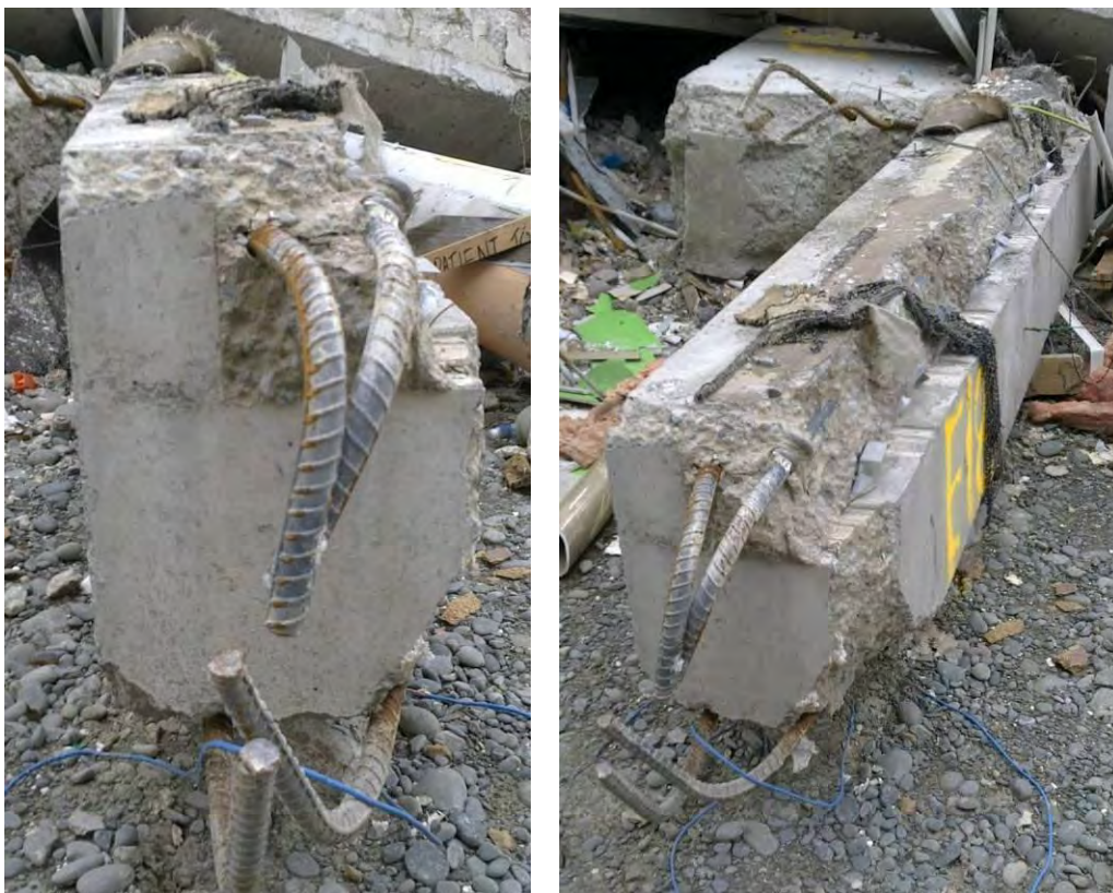
Figure 13 - Item E18 Pre-cast edge beam north-west corner (DENG B22 Dwg S18 (Figure 67) (from left to right) (a) Smooth form finish at attachment to column 4A (DENG Detail I Dwg S19 (Figure 70)); (b) No starter bar reinforcing steel extended from this pre-cast beam into slab. This was consistent with what was shown on the Drawings (DENG Section 4 Dwg S15 (Figure 66).
