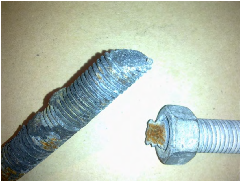
Figure 37 - M20 Drag Bar Bolts (Portions shown are from two different bolts) (left to right) (a) Grey portion with smooth diagonal end had epoxy residue from slab indicating it was cut this way prior to installation; (b) Necked and dimpled fracture surface at underside of bolt typical of direct tensile fracture in threaded rods.
