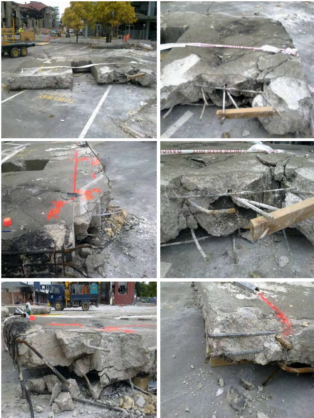
Figure 20 - Line 1 South Wall Level 4 to Level 5 (Item E4) (clockwise from top left) (a) Outer face with east pier on right with severe shear damage, and timber formwork remnant; (b) and (c) Charring on fractured concrete surfaces prior to deconstruction; (d) Top west corner showing saw-cut on top edge from deconstruction; (e) Top east corner showing smooth construction joint at interface with pre-cast beam B15 (DENG Dwg S18 (Figure 67)) and fire charring to spalled eastern edge; (f) View from east to west of top east corner construction joint notch.
