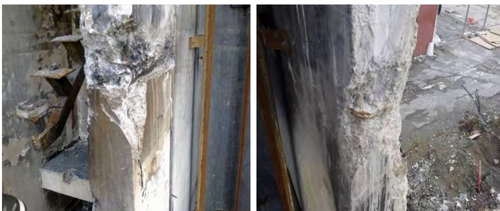
Figure 34 - Level 2 Lift Well Wing Walls Grid D and D/E (left to right) (a) 20 mm hole in end where a reinforcing bar has pulled out of wall. 200 mm thick construction joints in wall at slab level; (b) No reinforcing steel attachment into the east wing wall at Level 2
