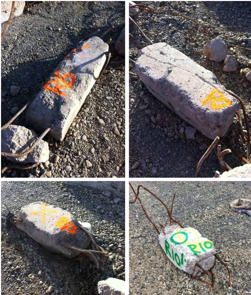
Figure 56 -400 x 300 mm Rectangular Columns (from left to right and top down) (a) tR6 base at far end connected by reinforcing to (b) tR7 below, with beam-column joint failure; (c) tR10 remnant; (d) tR10' remnant
