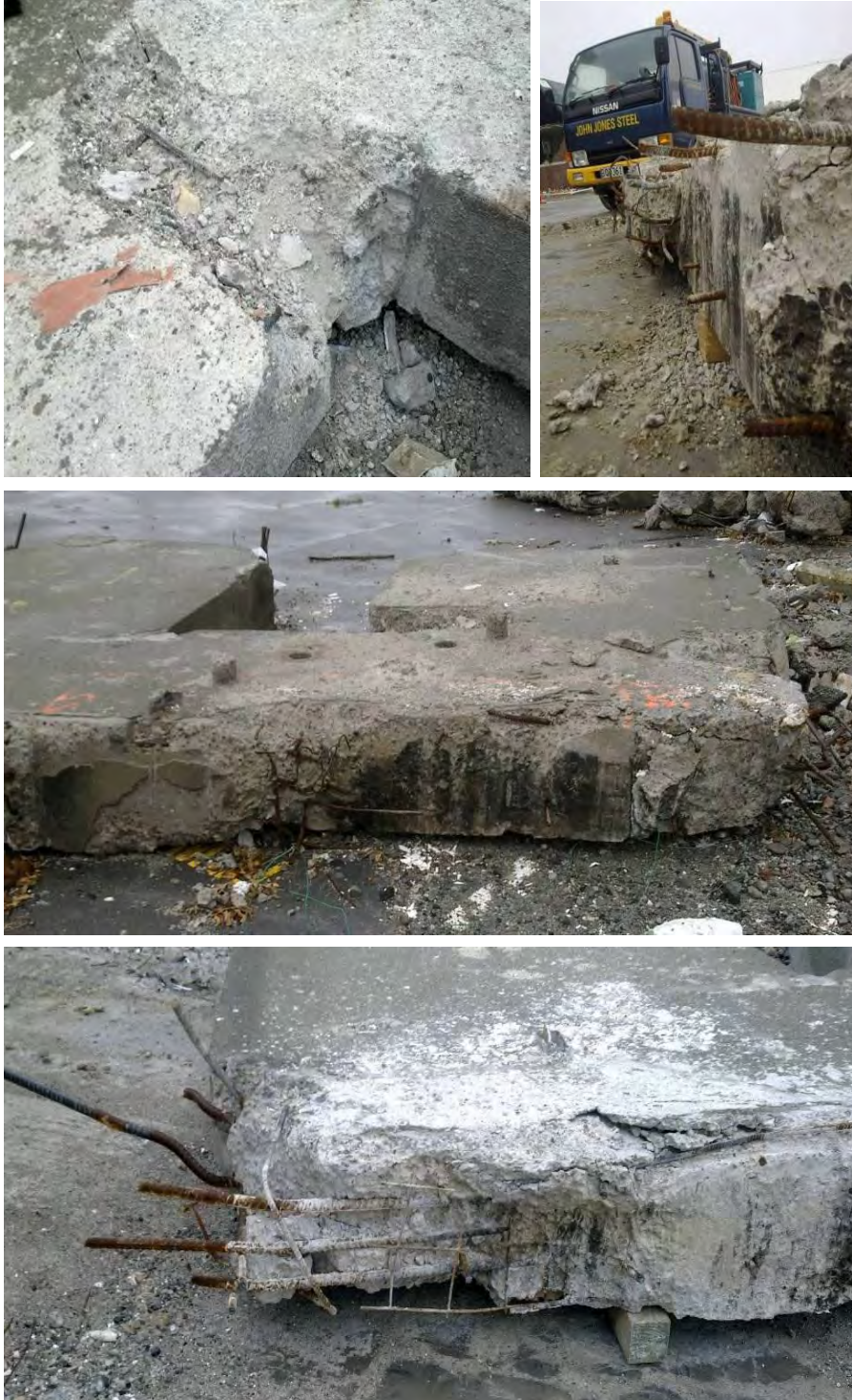
Figure 22 - Line I South Wall Level 5 to Level 6 (Item E5) (clockwise from top left) (a) Crumbly concrete at door edge of west pier able to be dislodged by boot; (b) Smooth and charred construction joint on top west surface looking east; (c) Charred construction joint above west pier. Door sill on left; (d); Top east corner with fractured top 3-H24 bars. Floor 664 mesh exposed.
