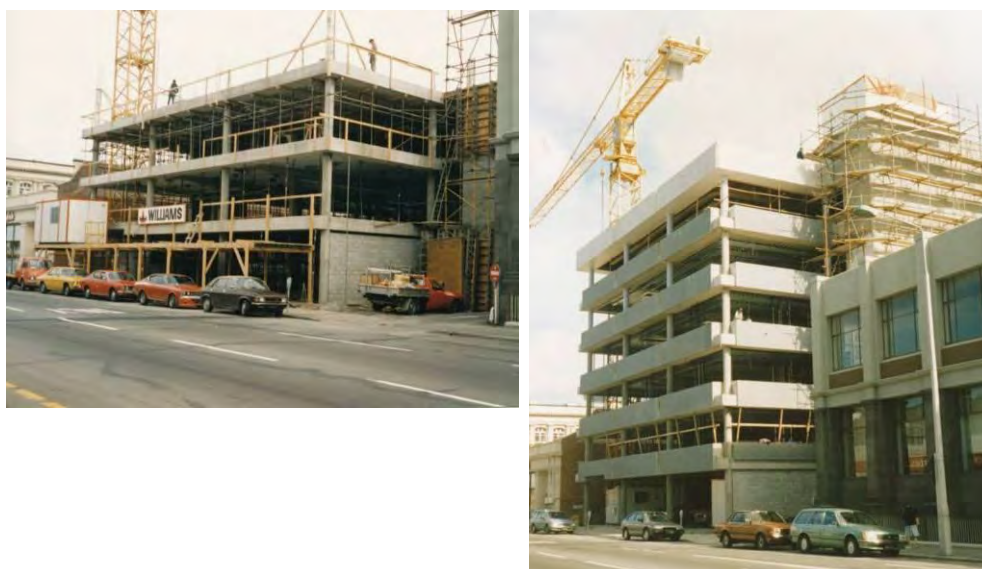
Figure 45 - CTV Building under construction (left to right) (a) May 1987 with floors cast up to Level 4; (b) October 1987 with roof on and pre-cast spandrel panels attached; Columns C21 to C23 had not been built at that time in the northeast corner closest to camera.
