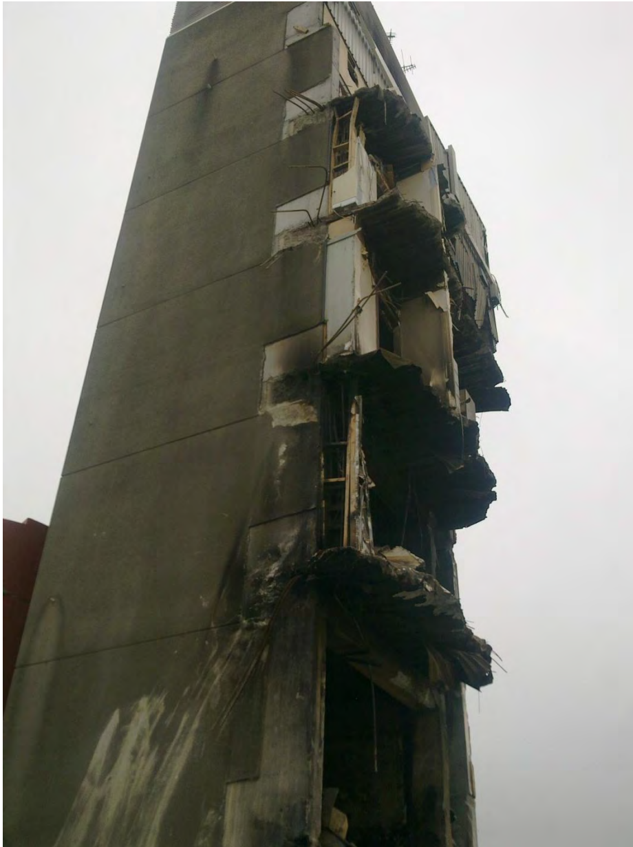
Figure 2 - West face of North Core (Wall Line C) showing the locations where the Line 4 beams had connected into the wall at Levels 3 to 6 without the bottom bars being developed into the wall as specified.
