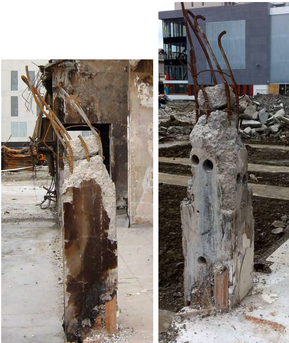
Figure 47 – Locations of concrete cores taken on site for testing on column C18 on Line 4, adjacent to wall D/E
