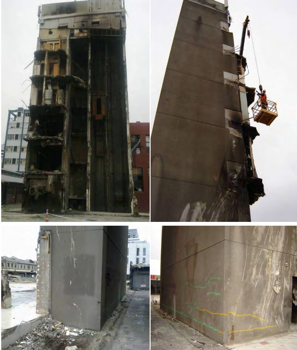
Figure 25 - Line 4 to 5 North Core (DENG Dwg S15 (Figure 65)) (clockwise from top left) (a) South face after site cleared with lift shaft for two cars on right, stair well in middle and amenity rooms on the left; (b) West face; (c) West and north face at Grid C/5 corner Level 1 to 2 with horizontal flexural cracks and construction joint identified by paint; (d) East face with column C18 remnant at far left
