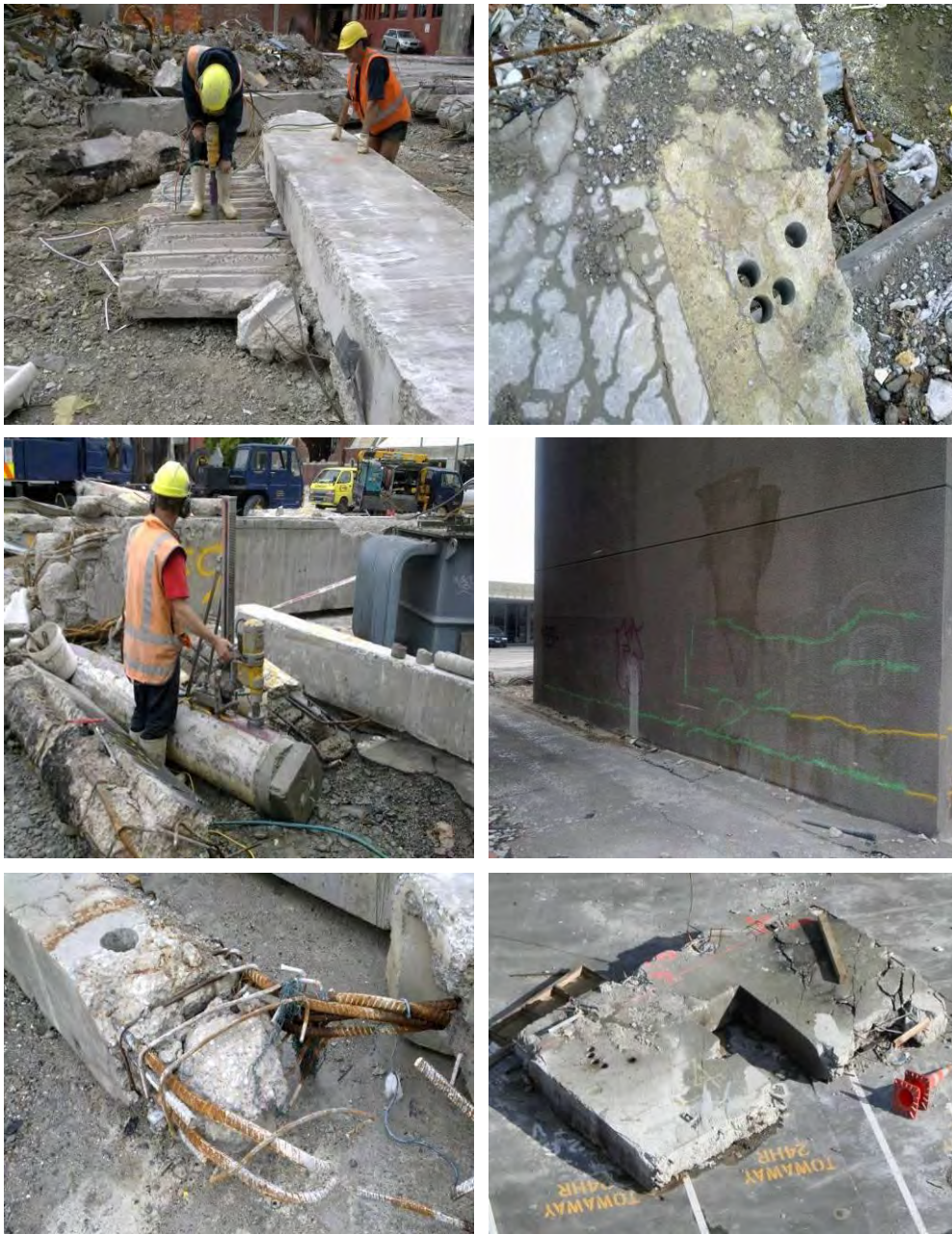
Figure 46 – Locations of concrete cores taken for testing (clock-wise from top left) (a) Slab attached to Line 1 or 4 perimeter shell beam (Item E23) (b) Slab attached to Line 4 perimeter shell beam (Item E14); (c) Line 5 shear wall through stair well at Level 1; (d) Line 1 South wall Level 4 to 5 (Item E4); (e) Pre-cast log beam from Line 2 or 3; (f) Level 6 400 mm diameter column (Item E25)
