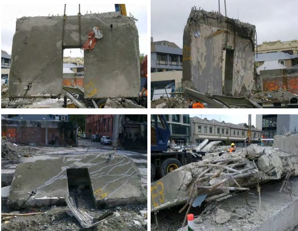
Figure 18 - Line 1 South Wall Level 3 to Level 4 (Item E3) (clockwise from top left) (a) Outer face; (b) Inner face; (c) Damaged top east corner; (d) One way diagonal cracks running from bottom west to top east side marked by paint on outer face.
