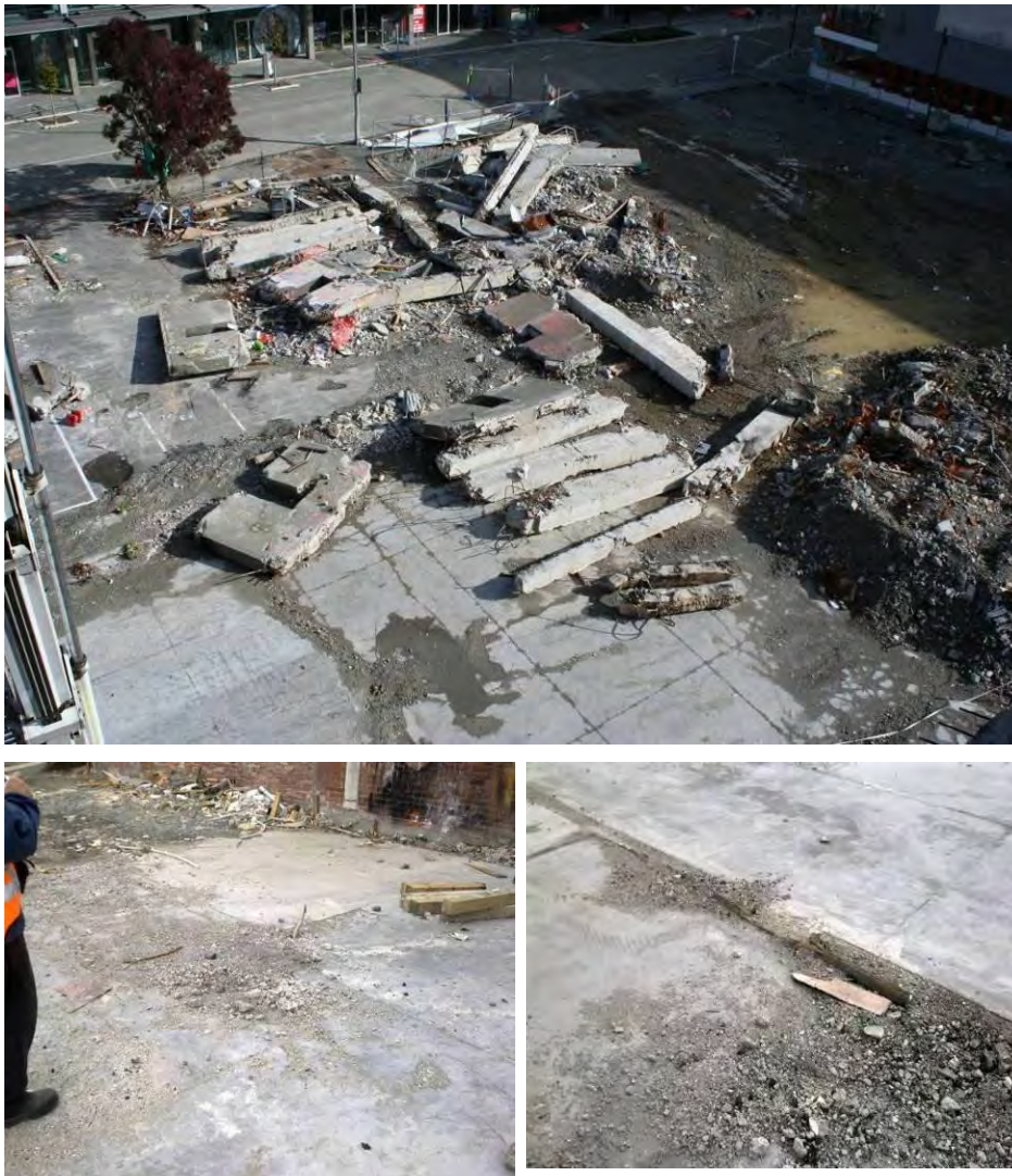
Figure 4 - Ground floor Level I slab on grade (clockwise from top) (a) View from snorkel of debris and western portion of Level I slab on grade; (b) Slab in northwest corner with column reinforcing protruding; (c) Ramp formed in concrete overlay in front of Line 4 lift core walls.
