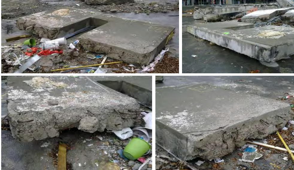
Figure 24 - Line 1 South Wall Level 6 to Roof (Item E5A) (clockwise from top left) (a) Outer face; (b) Top surface at roof; (c) East pier with saw-cut from de-construction; (d) West pier at construction joint
