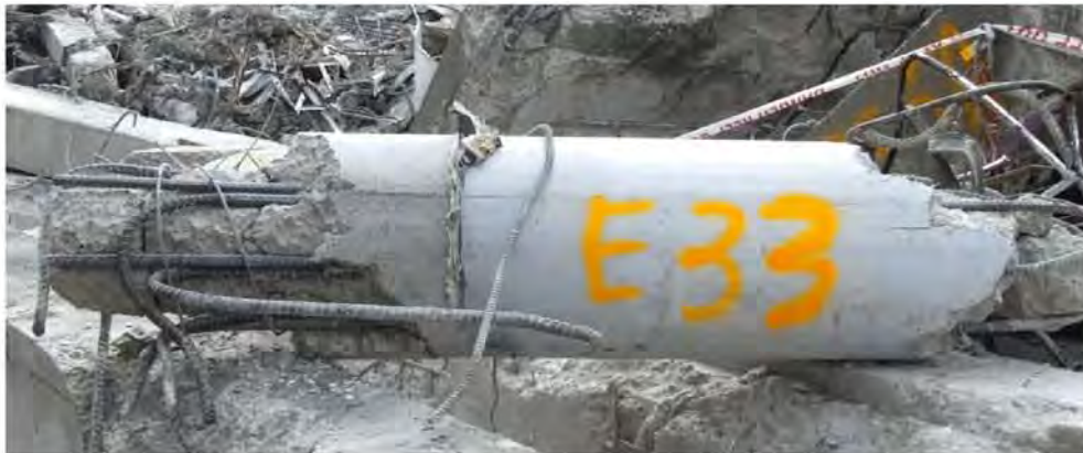
Figure 89 - Perimeter 400 mm diameter column with spalled base and bar lapping zone at left unpainted portion that would have been located at Spandrel Panel infill areas.
