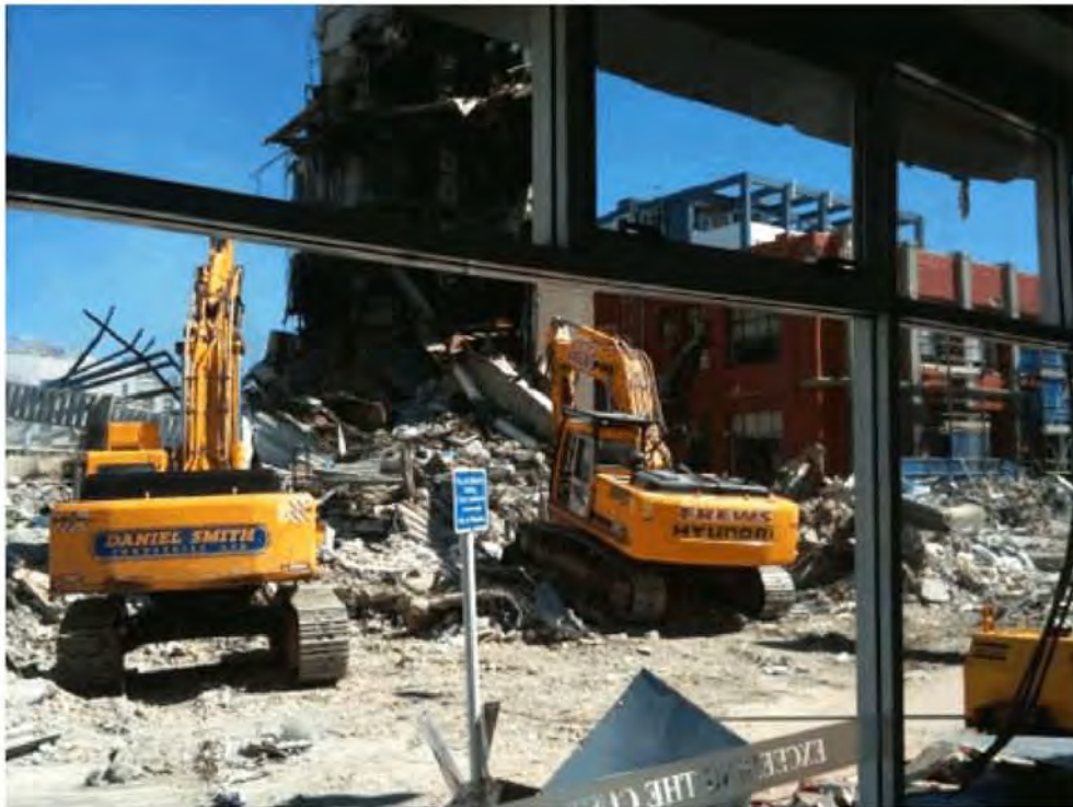
Figure 85 - Debris being cleared from Madras Street face.
