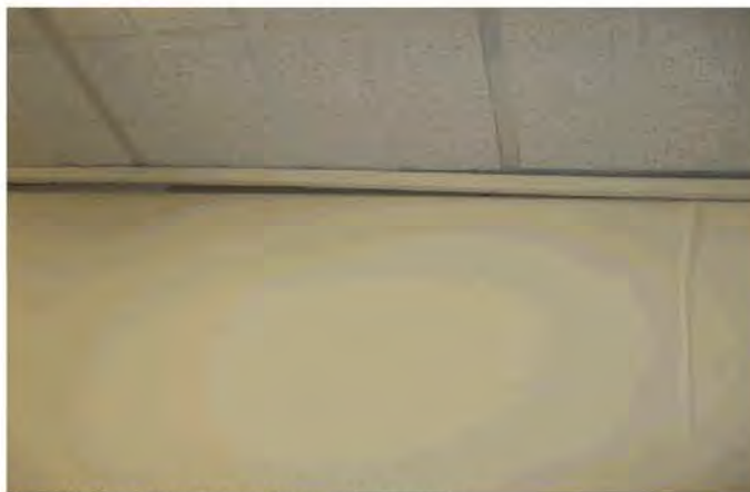
Photo 14 Cracked wall lining and damaged ceiling coving.
