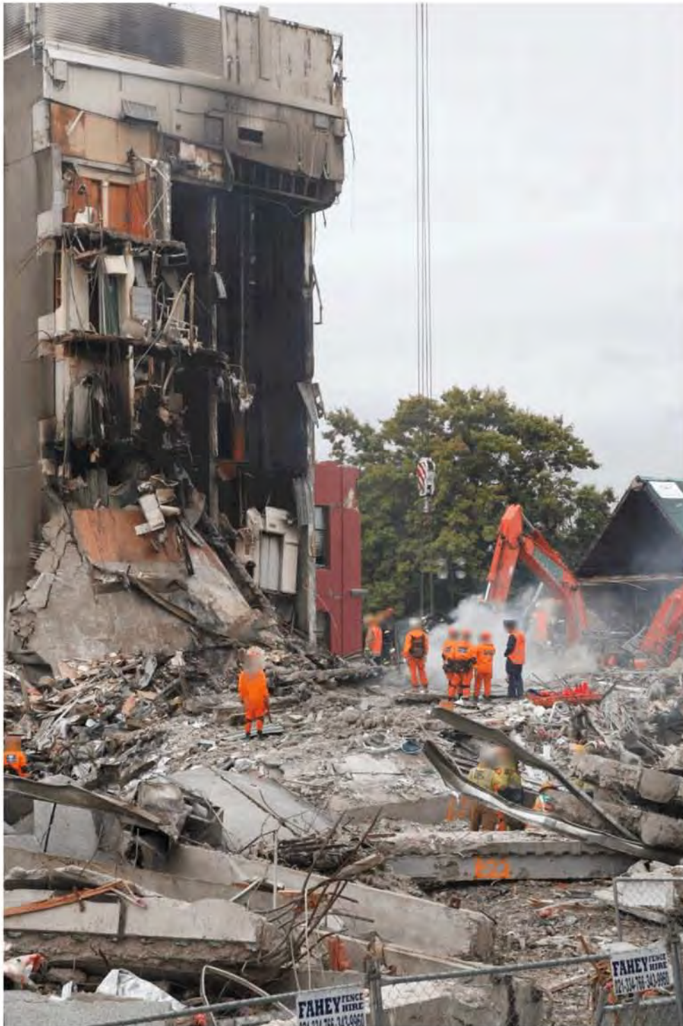
Figure 97 – View from southwest of North Core. The Level 4 slab can be seen lying diagonally against the North Core.
