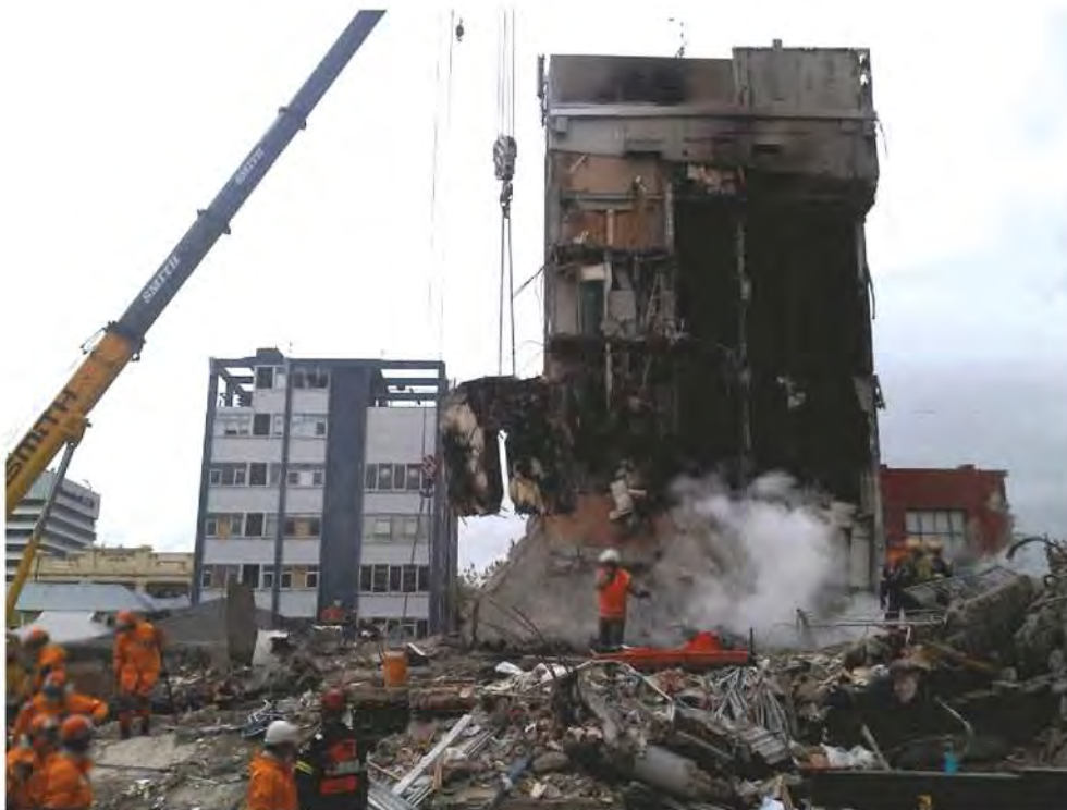
Figure 91 - Portion of Line 1 South Wall being lifted out by crane.. The Level 6 slab in front of North Core has been removed for safety reasons.
