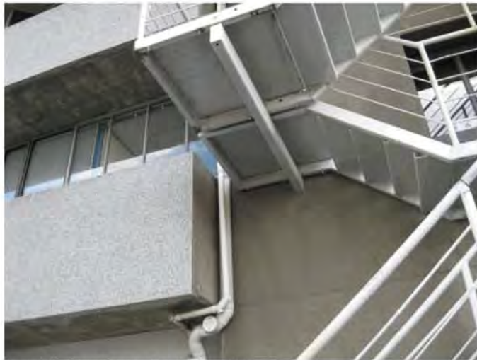
Photo 6 Spalling of plaster off ends of spandrel panels.
