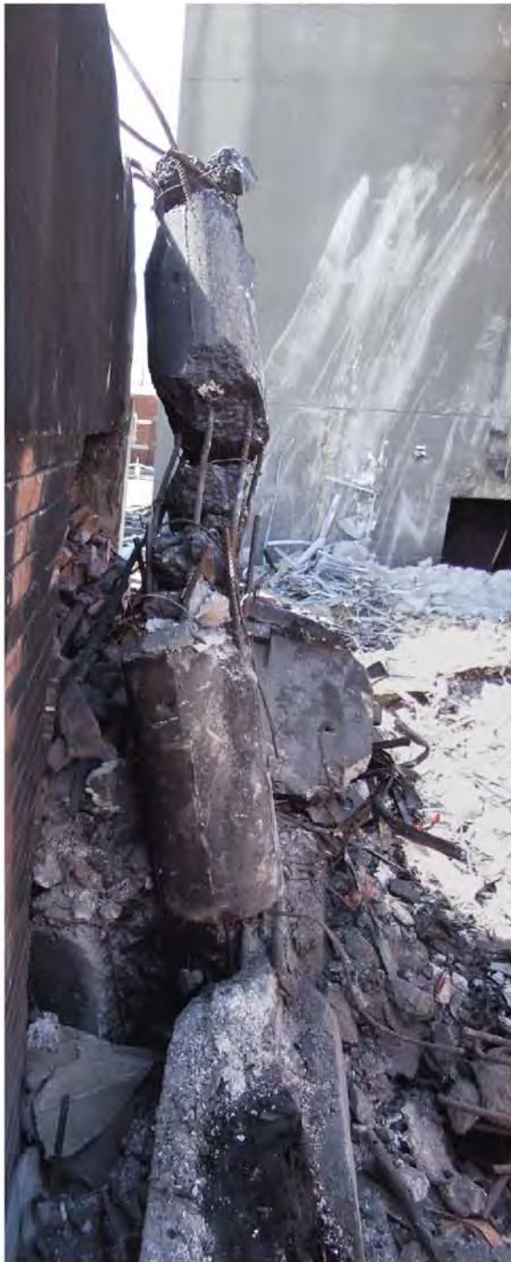
Figure 101 - Line 4 / B column with B22 precast log beam in foreground and B23 shell beam at rear. No hinging is apparent at the base of the column compared to the perimeter column Item E33.
