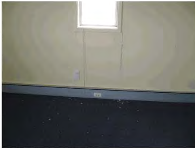
Photo 12 Cracking in linings under window.
