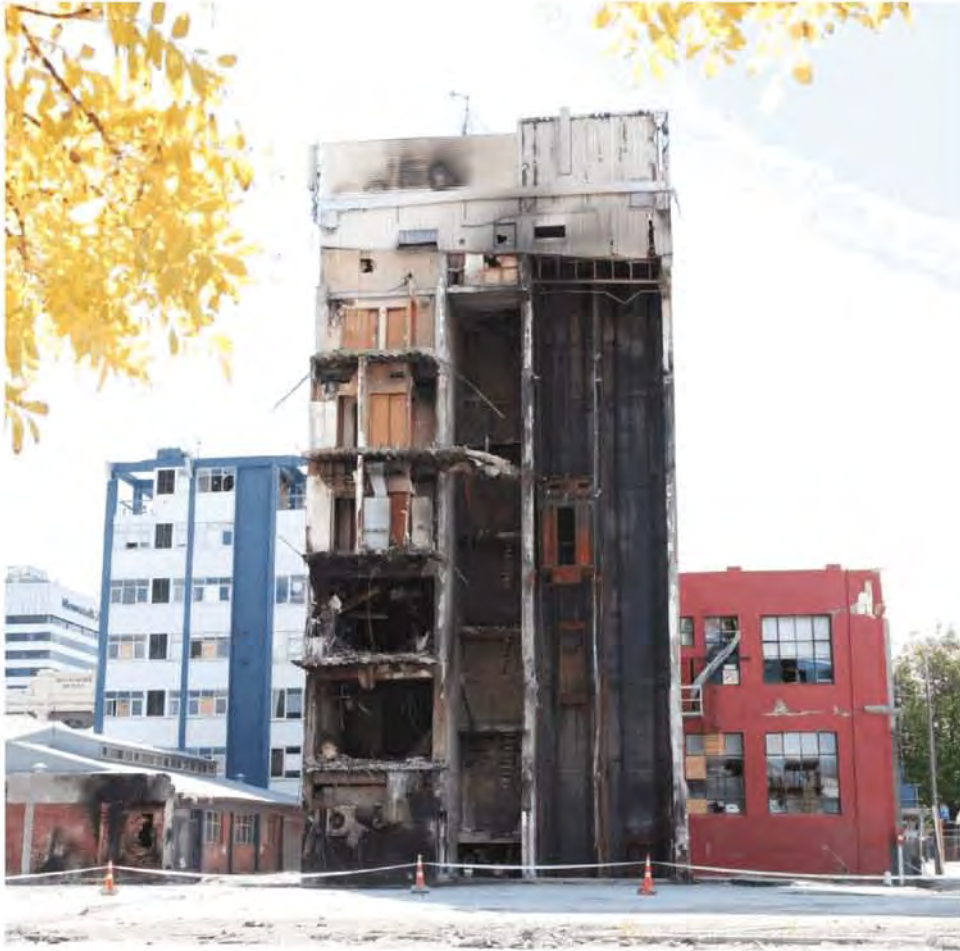
Figure 104 - All debris removed leaving the Level 1 slab on grade and remnants of the North Core.
