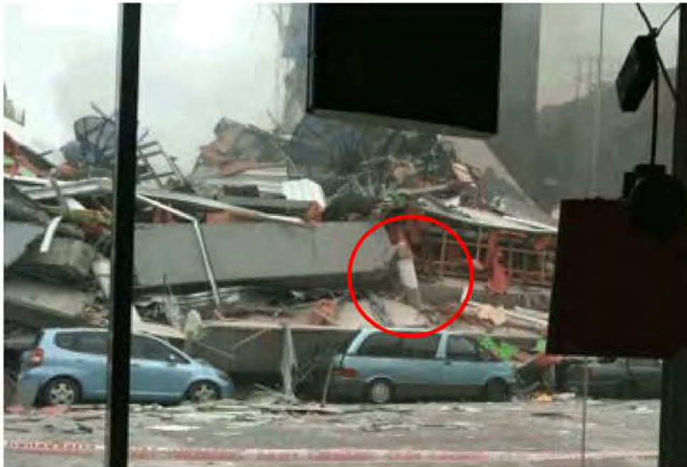
Figure 79 – View from looking west across Madras Street. A Line F/3 column is highlighted showing conical fracture in the painted portion above unpainted portion which had been enclosed by Spandrel Panels.
