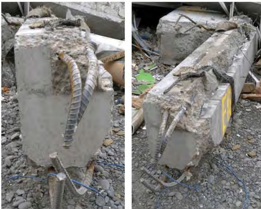
Figure 108 - Item E18 Pre-cast edge beam north-west corner (DENG B22 Dwg S18 (from left to right) (a) Smooth form finish at attachment to column 4A (DENG Detail 1 Dwg S19); (b) No starters (reinforcing bars) from pre-cast beam into slab to prevent the profiled metal deck slab pulling away (DENG Section 4 Dwg S15). If roughened these joints may have slowed down development of progressive collapse.
