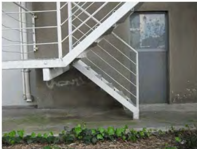
Photo 2 Cracking in south shear wall (not visible in photo) under fire escape landing
