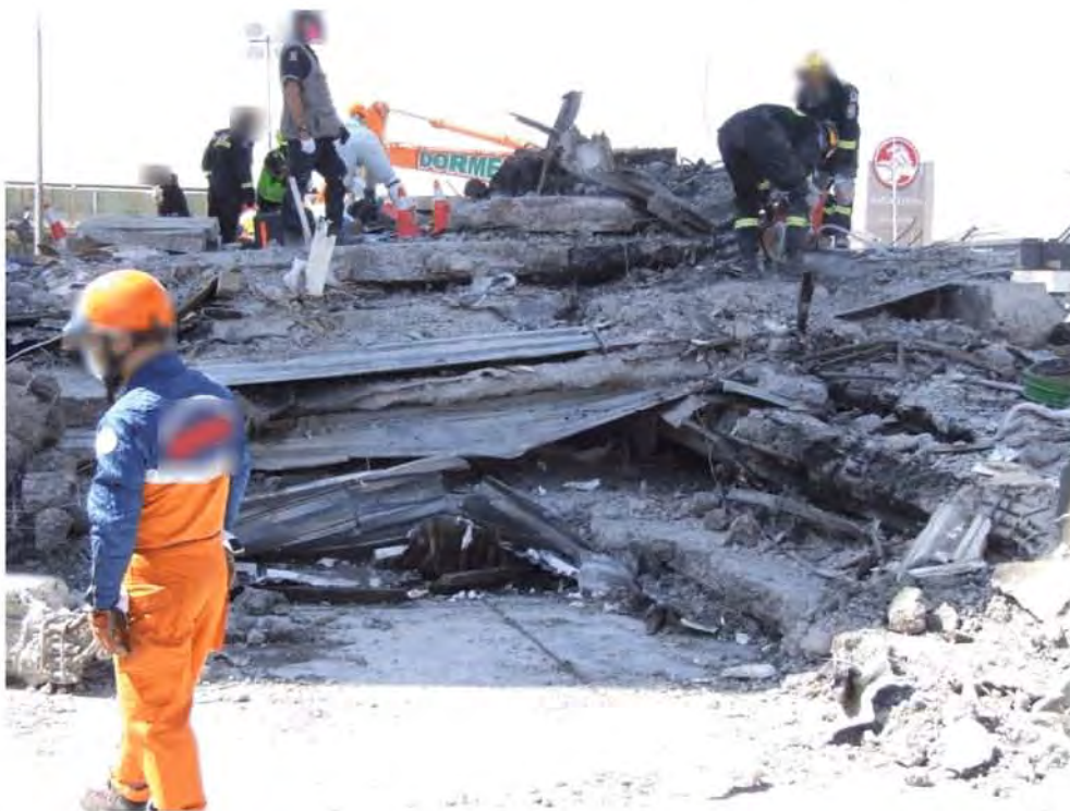
Figure 98 - Line 2 beams lying rotated northwards.
