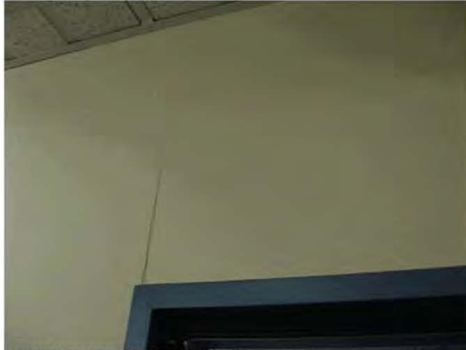
Photo 11 Cracking in linings over door head
