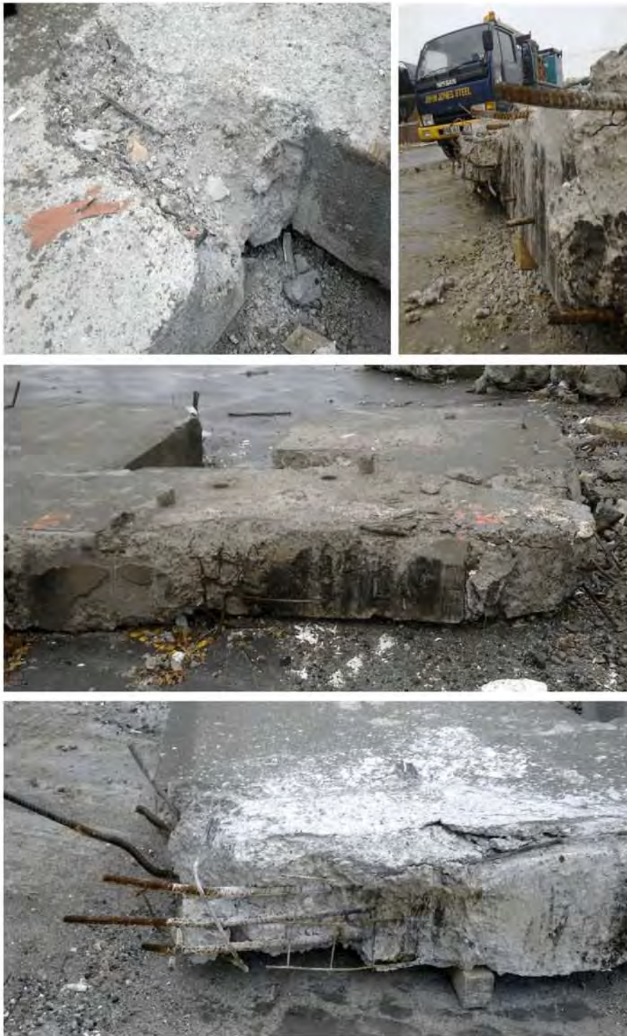
Figure 112 - Line 1 South Wall Level 5 to Level 6 (Item E5) (clockwise from top left) (a) Crumbly concrete at door edge of west pier able to be dislodged by boot; (b) Smooth and charred construction joint on top west surface looking east; (c) Charred construction joint above west pier. Door sill on left; (d); Top east corner with fractured top 3-H24 bars. Floor 664 mesh exposed.
