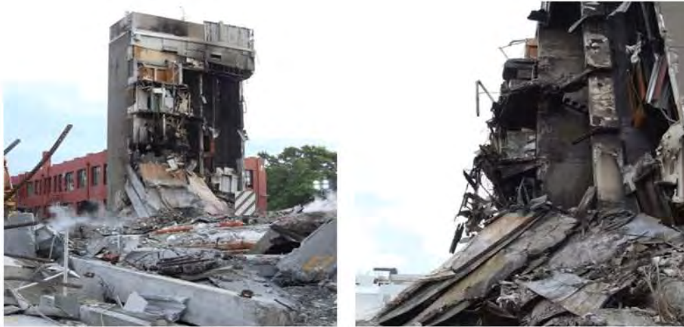
Figure 95 – View of North Core showing Level 4 slab lying diagonally on top of Level 3 slab. This indicates that the Level 3 and 4 slabs lost their vertical support on Line 3 prior to breaking away from the North Core.
