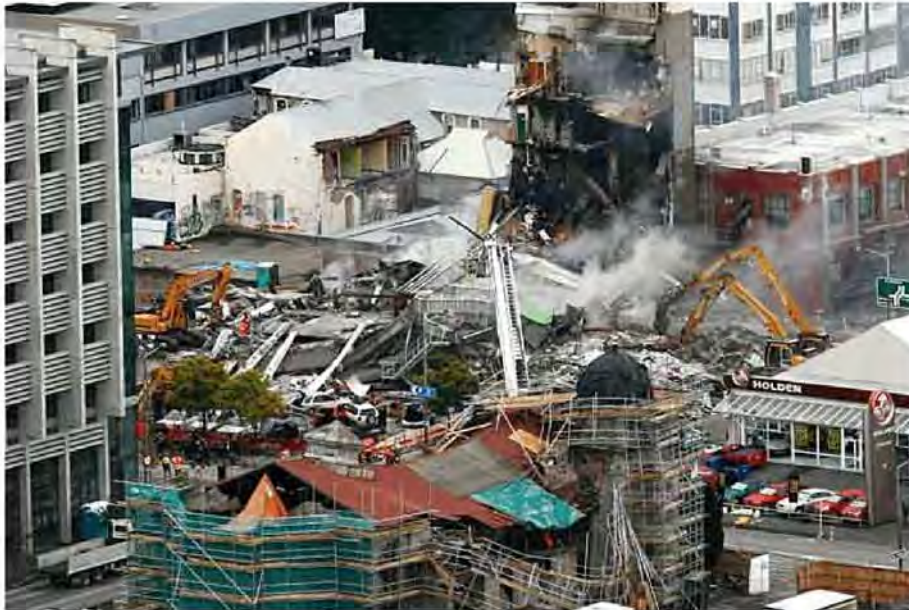
Figure 80 - Aerial view from southeast with debris being removed by heavy machinery. Fire has blackened the North Core. The Samoan church is damaged in the foreground (Dominion Post).
