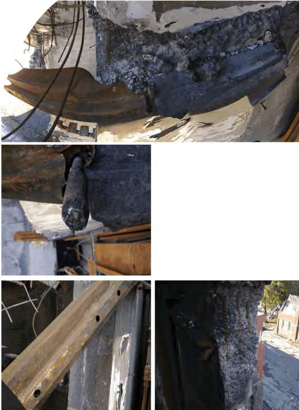
Figure 115 - Level 5 Lift Well Wing Walls Grid D and D/E (anti-clockwise from top) (a) the Drag Bar consisted of a 150x150x10 L steel angle with a 51 x 3.2 SHS welded to it; 4-M24 anchors were epoxied into the wall and 6-M20 threaded anchor rods 350 mm long were epoxied into the slab at the profiled metal deck rib. 3-M20 threaded rods remained upright on the Grid D Drag Bar. The 51x3.2 SHS had fractured in bending and tension at the bolt hole adjacent to last bolt into wall and twisted with the slab; This shows that the slab that had been fixed to the Drag Bar had rotated downwards as the column on Line 4 D/E collapsed, (b) Epoxy grout can be seen around the threaded anchor rod that had been in the slab; (c) The Drag Bar is bent downwards and holes where 3-M20 threaded anchor rods had been can be seen; d) On Wall D/E a 150x75x10 L steel Drag Bar was still fixed into the wall D/E with 5-M24 threaded rod anchors. The end of the Drag Bar had been gas cut during deconstruction.
