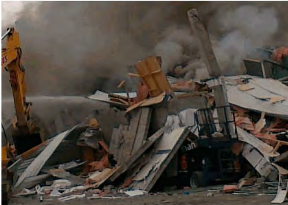
Figure 153 - West wall on Line A at southwest corner shortly after the collapse.
