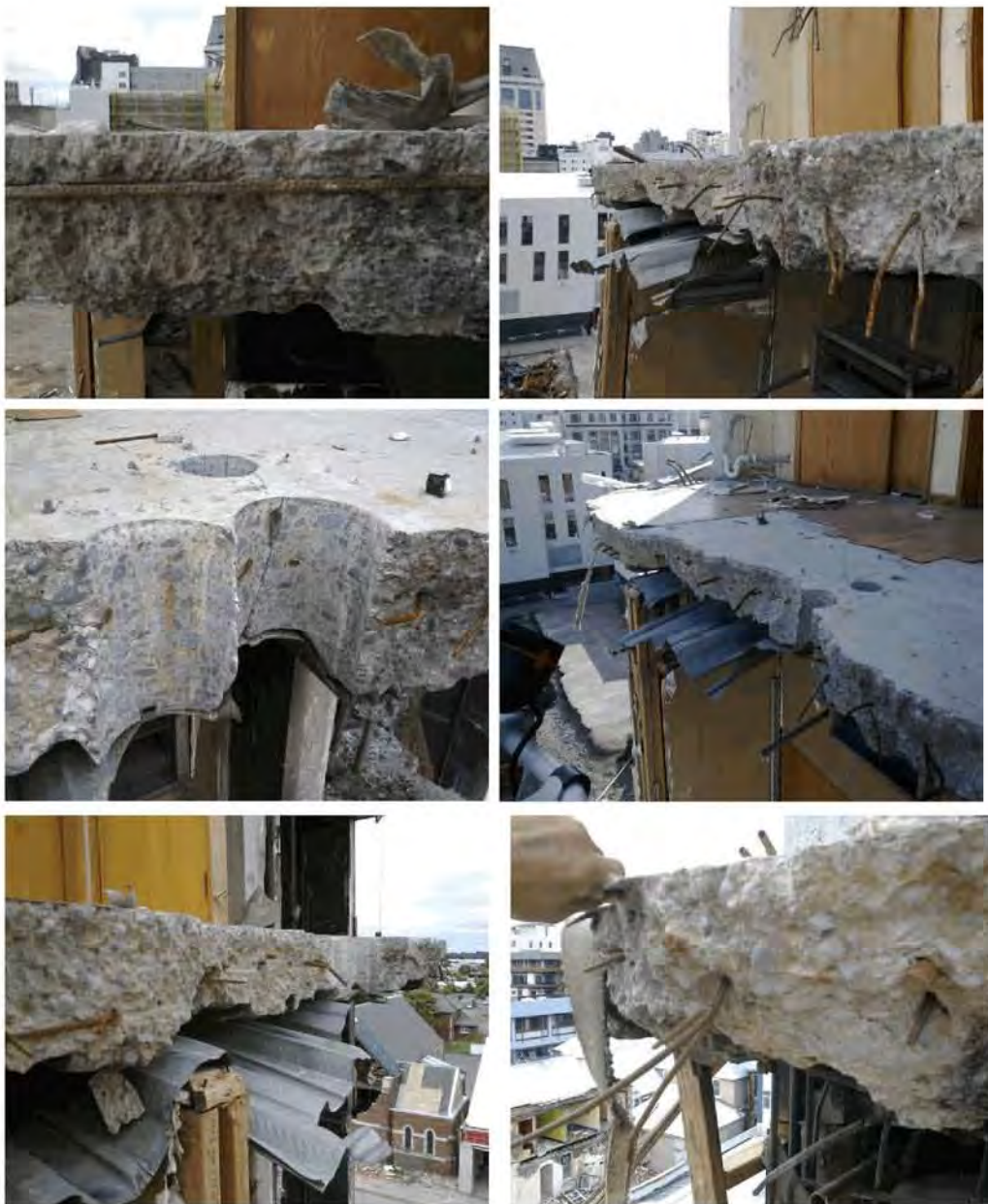
Figure 114 - Line 4 Core Wall Slab Remnant at Level 6 amenity area (clockwise from top left) (a) Slab edge on stairwell wall looking west with HI2 saddle bar exposed and ends of mesh below it; (b) Vertical concrete fracture surface with reinforcing mesh fractured; (c) Slab looking west with cores cut in floor for amenities; (d) Fractured mesh angled downwards; (e) Fractured slab edge looking east. Torn metal decking aligned approximately with concrete fracture edge; mesh at varying height within slab; (f) Cores for amenities at fracture edge can be seen and are a small proportion of the total fracture surface length.
