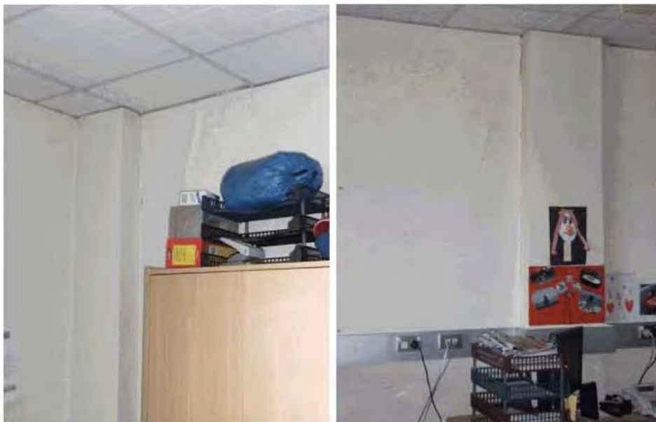
Figure 152 - Inside of the west wall at Level 2 after the 4 September 2010 Earthquake shows some damage to the linings.
