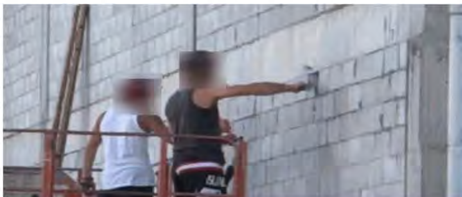
Figure 150 – Workers (including Eyewitness 16) hammering face of top course block away on west wall near Line A / I corner column. This indicates hollow blocks occurred in the top course and no separation joints on the outer face of the masonry.
