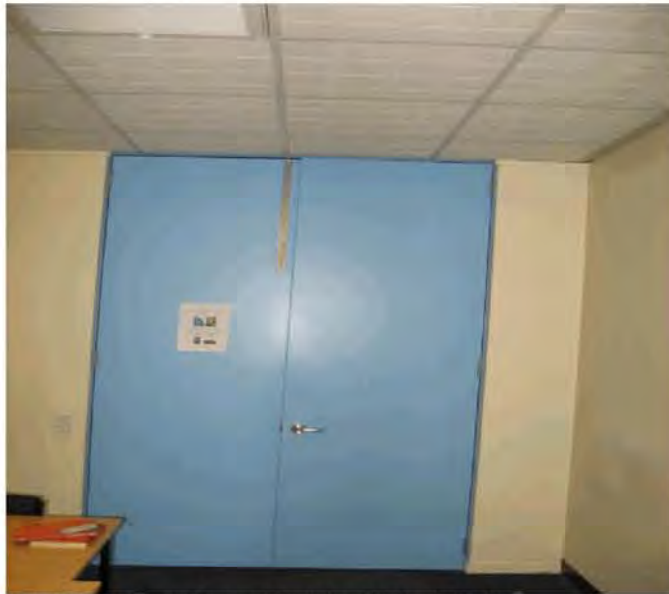
Photo 13 Racked second floor partition wall and binding double doors.
