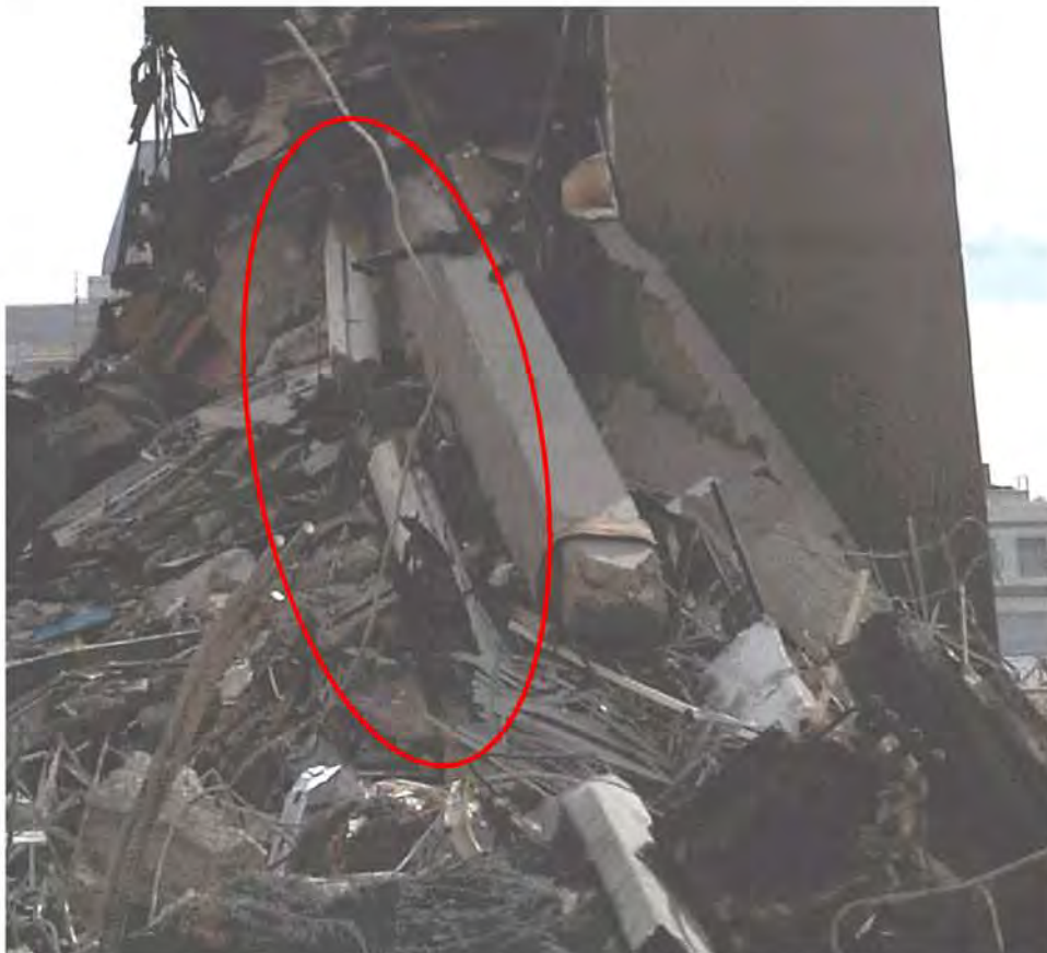
Figure 96 - North Core column 4 D/E highlighted amongst the debris. Hinging can be seen above and below the beam column joint.
