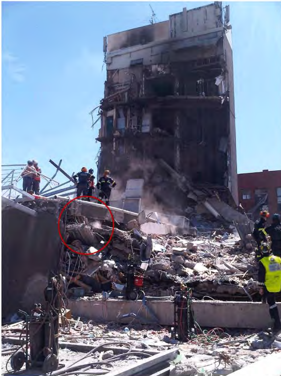
Figure 90 - View from Cashel Street east side of Line 1 with Line 1 South Wall lying on debris at left; trapezoidal end profile of floor slabs laying on top of each other in foreground; A portion of floor slab highlighted, appears to be still in contact with the South Wall at Level 2. Remnants of North Core slabs and the collapsed column on Line 4 D/E can be seen at the rear. The Level 6 slab in front of the lift well can be seen still suspended in mid-air by its Drag Bars connected at Walls D and D/E, even after loss of support from column 4 D/E.
