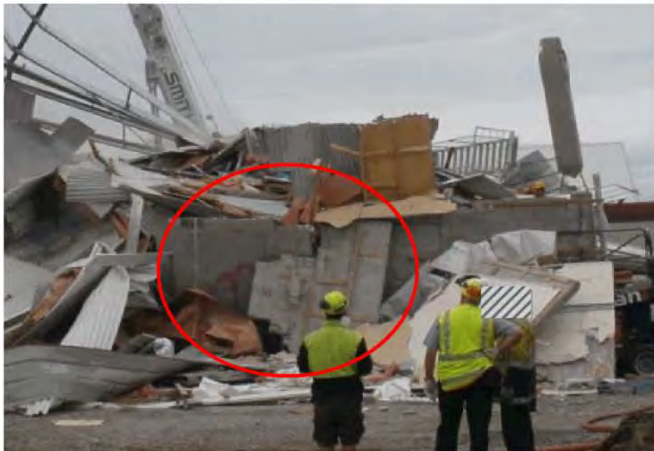
Figure 154 - West wall shortly after collapse. The corner Grid 1/A column is still standing and the wall panels have broken free in panel sections in places. The edges of the panel section are square consistent with the design drawings. Diagonal fracture of the masonry infill that has fallen outwards from level 2 is highlighted. This indicates that the infill masonry above Level 2 fully developed its shear capacity prior to the collapse and therefore affected the response of the structure to the February Aftershock.
