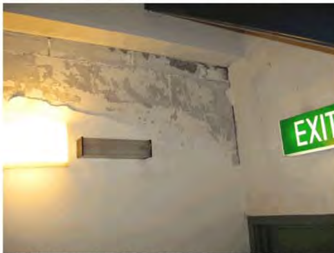
Photo 8 Spalling gypsum plaster off non-load bearing concrete block wall in stairwell.
