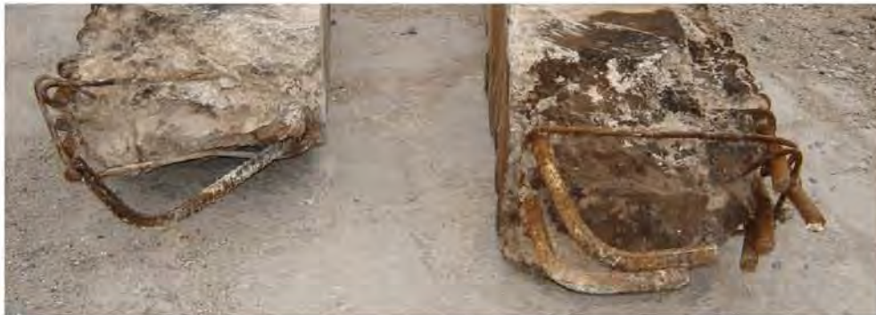
Figure 107 - Interior Pre-cast Log Beams from Line 2 and 3 (DENG Section 3 Dwg S15) showing smooth concrete formed for beam-column joint, and bottom hooked bars that have pulled out of beam-column joints without any obvious straightening;
