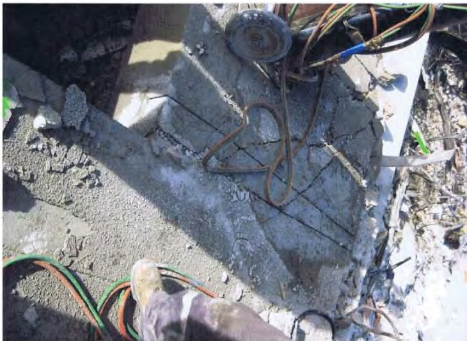
Figure 94 – Line 1 South wall at Level 4 showing severe diagonal cracking in east panel.
