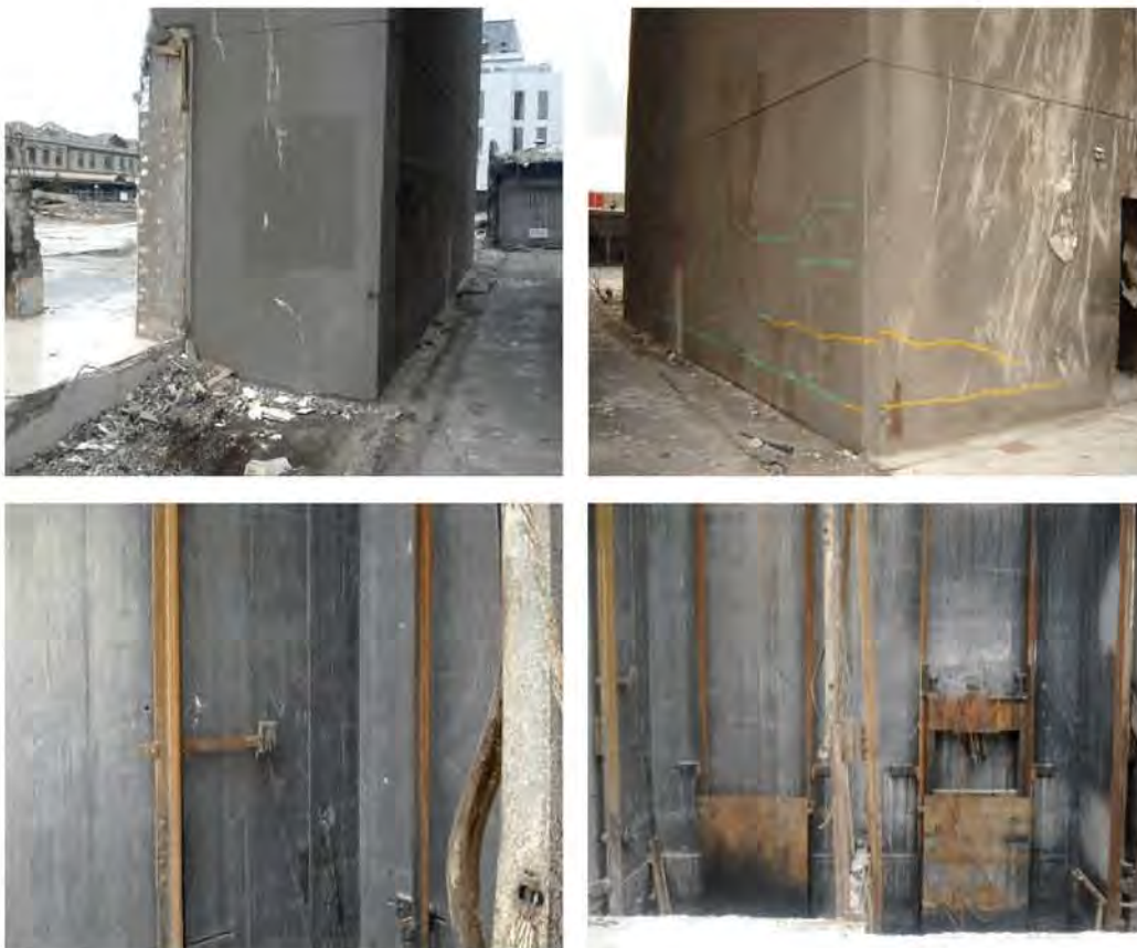
Figure 113 - North Core cracking (clockwise from top left) (a) No obvious cracking on Line D/E wall; (b) Horizontal flexural cracking on west and north west face of Line 5 wall and north end of Line C wall at Line C/5; (c) Fine two-way diagonal cracking on the inside faces of Level 1 to 2 Line 5; (d) and D walls in North Core.
