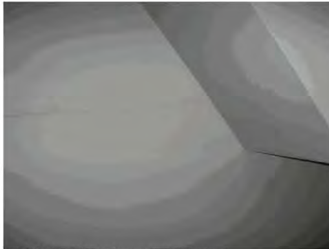
Photo 3 Cracking in floor level construction joints in stair well
