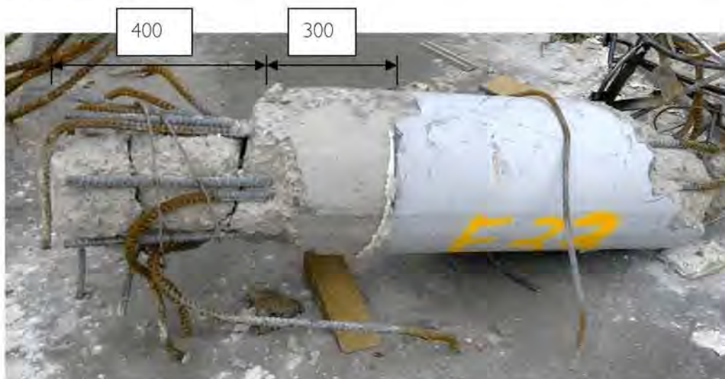
Figure 106 - 400 Diameter Exterior Column Item E33. (DENG C5 or C11, Dwg S15). Left end is bottom of column at floor level with concrete spalling over lapped vertical reinforcing. Horizontal cracking in core confined by R6 spiral which had fractured. The unpainted portion was protected by Spandrel Panels.. Right-hand end fracture occurred below beam-column joint.
