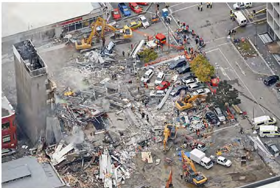
Figure 81 - Aerial view from northwest with heavy machinery removing debris. Water puddles on the vacant site may be due to fire fighting based on comparison with Figure 71 which showed no surface water immediately after the collapse (NZ Herald).
