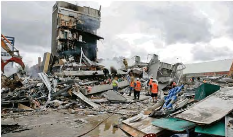
Figure 87 - View from Cashel Street with debris being cleared away from west wall.
