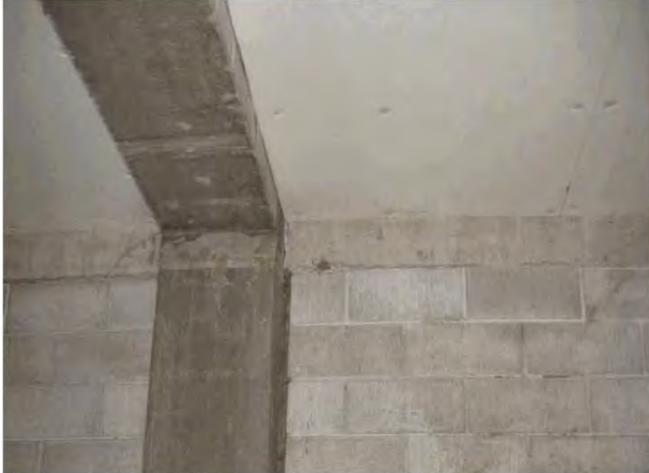
Figure 151 - Line A infill masonry wall adjacent to column with no obvious cracking after the 4 September earthquake. Flexible sealant is visible between masonry and column.
