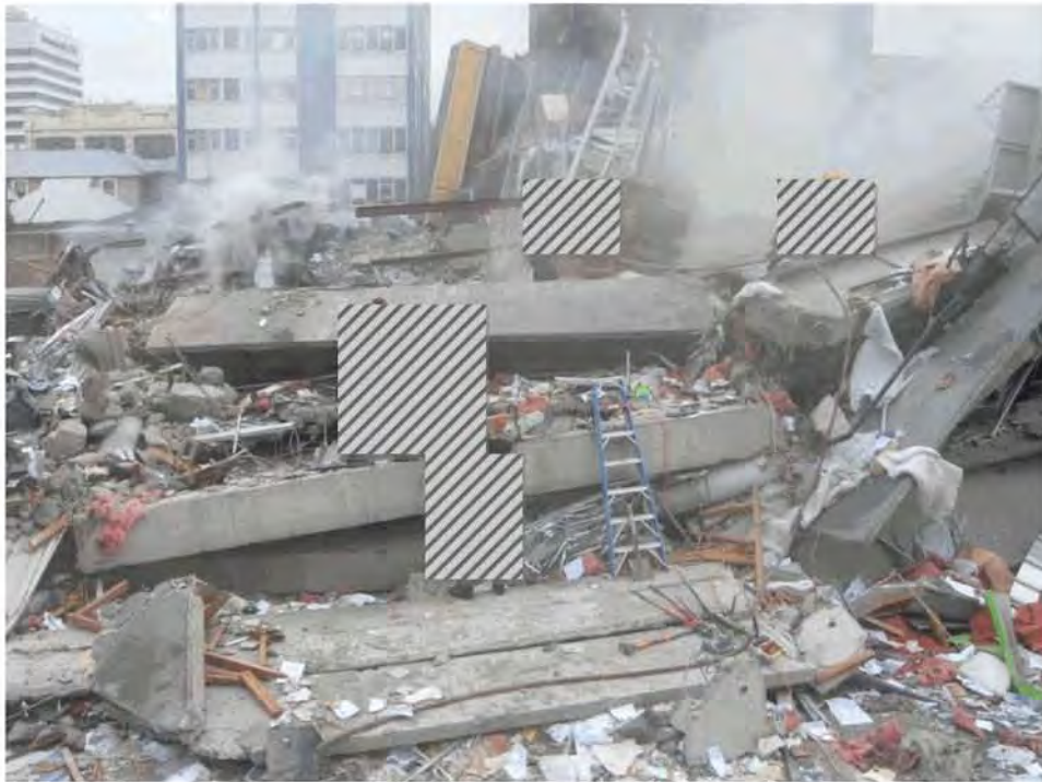
Figure 83 - Concrete Spandrel Panels, perimeter beams and columns on Cashel Street face (Line 1 / B-D).
