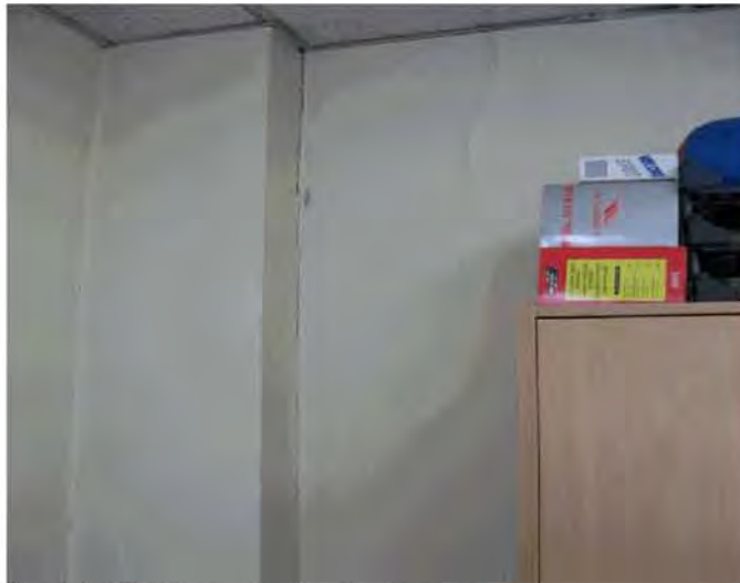
Photo 9 Partition lining damaged at junction with concrete column.
