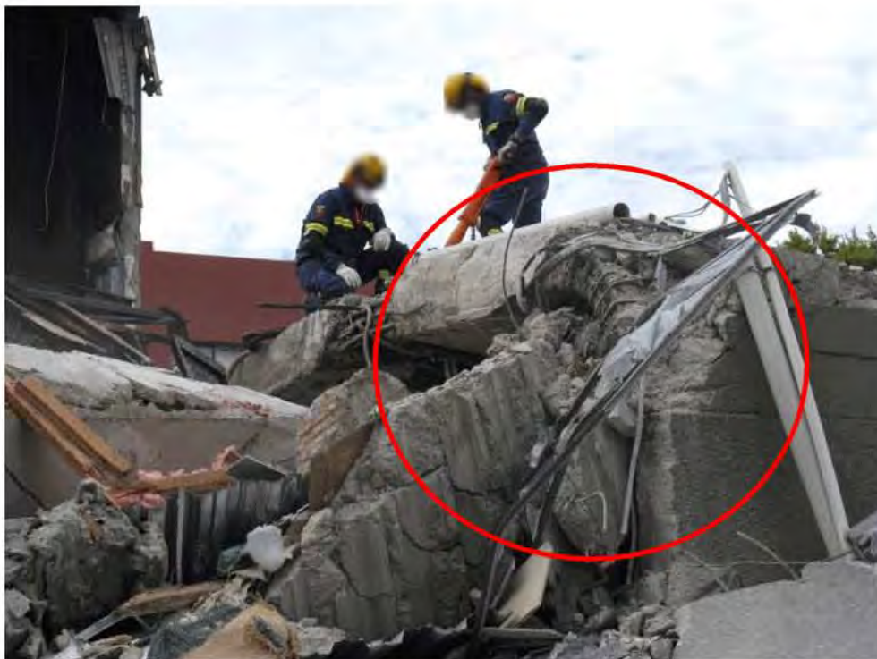
Figure 92 – Upper portion of South Wall being prepared for removal. A portion of slab can be seen highlighted in the foreground in contact with the South Wall on this side at Level 2. It may have forced the wall to pivot against it, preventing it breaking over at its base at Level 1.
