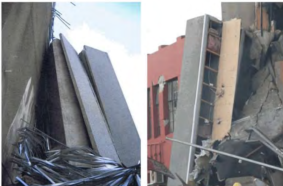
Figure 84 - Line 4 / B-C Spandrel Panels against tower wall, showing (left to right) a) View from north face; b) View from west showing timber framing for wall linings.
