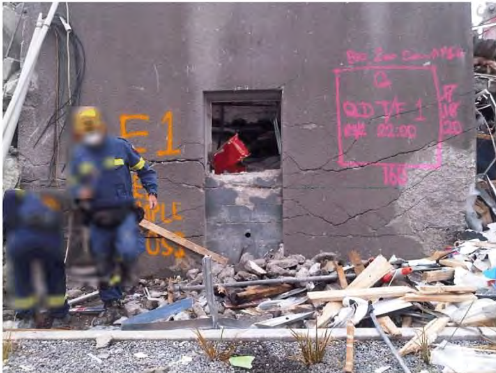
Figure 93 - Line 1 South Wall at Level 1 showing masonry in-fill at door opening, in-plane flexural fan-like cracking and spalling of concrete at right (east) end. A portion of profile slab can be seen end on through the opening
