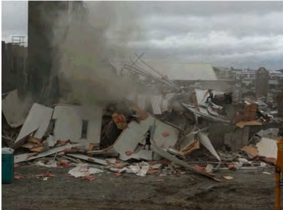
Figure 71 - West side of building with North Core partially obscured by smoke, prior to heavy machinery removing debris. No liquefaction evident.
