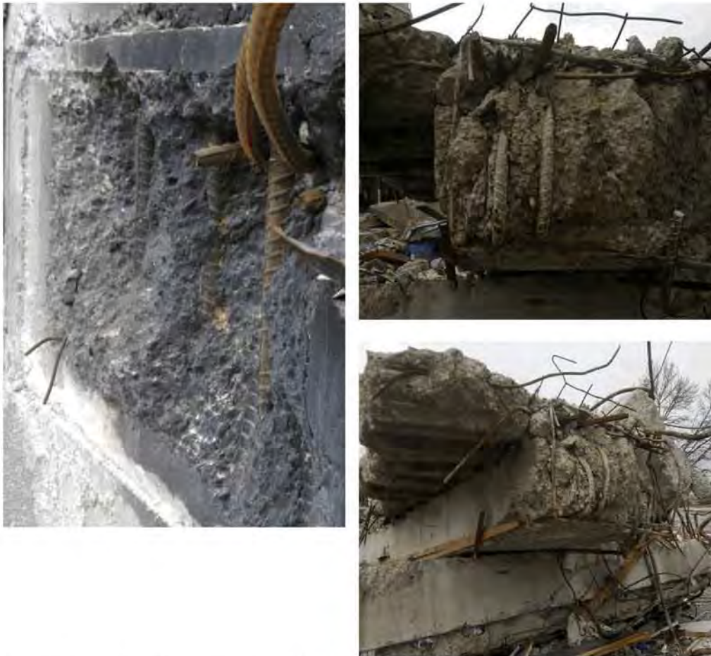
Figure 105 - Precast shell beam (Item E14) from northern face Grid 4, west side of North Core (DENG B23 Dwg S18). (clockwise from top right) (a) to (b) Fractured slab outstand remnant at east end from which slab concrete cores were extracted. The bottom H24 bars from shell beam have been turned back into the concrete infill rather than embedded in shear wall as specified (DENG Detail 5 Dwg S19). Notice the bar imprint on wall at the connection seen in (c) at Level 4 and at Level 3.. This meant that these beams would not have performed as intended.
