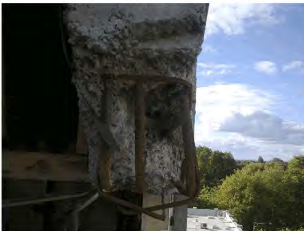
Figure 116 - Lift Well Wing Wall D/E: Column D/E 4 Connection (DENG Dwg S14); 3 x 20 to 24 mm diameter holes can be seen where reinforcing bars from column have pulled out. The drawing shows that 4-H20 bars were required to be bent in to the wall.
