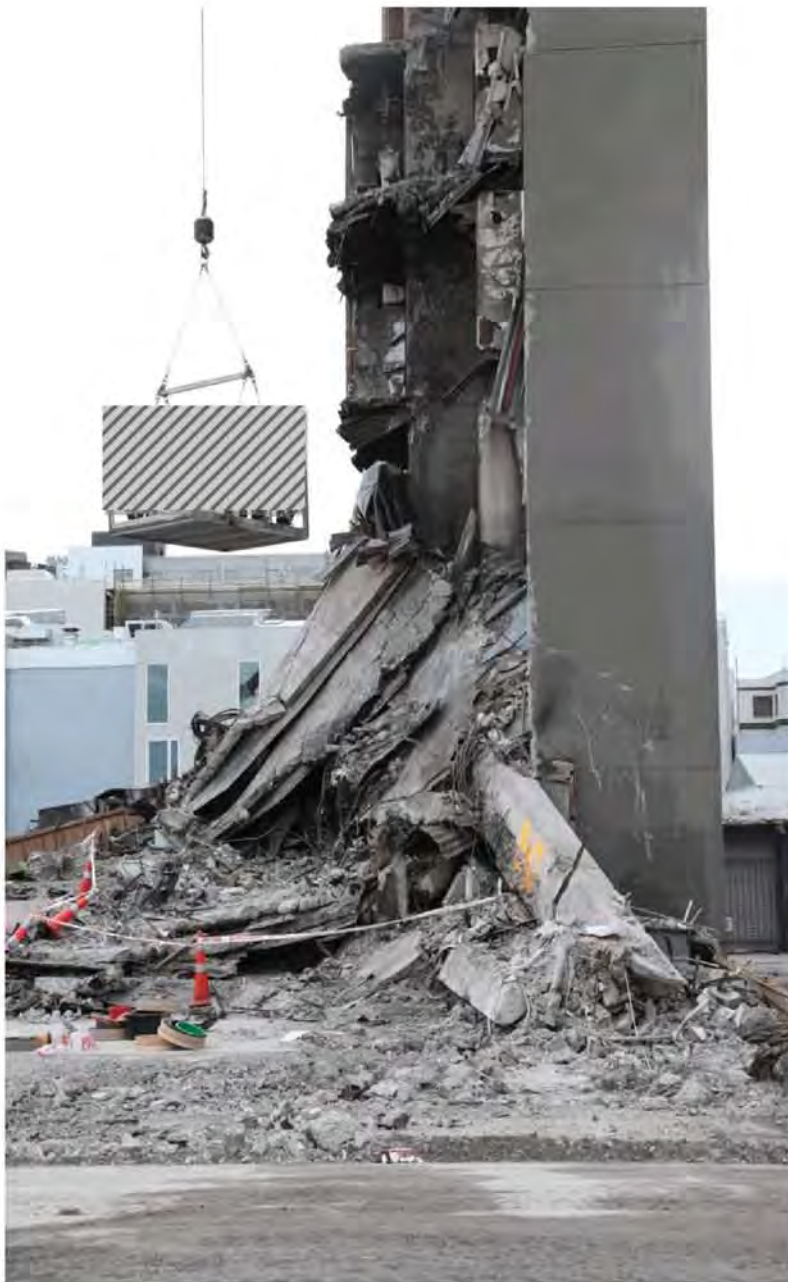
Figure 165 - North Core slabs leaning against the North Core showing that their collapse occurred after collapse of the Line 3 frame
