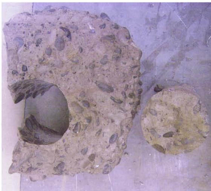
Figure 56 - Concrete from column on Line 4-D/E (C18) showing possible discolouration from silt.
