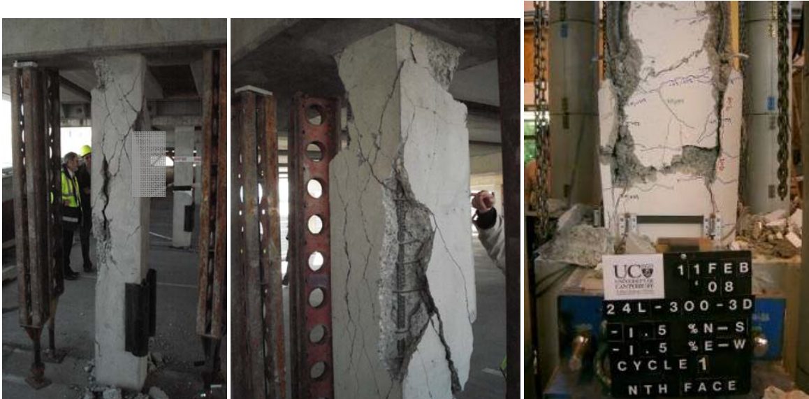
Figure 56: Severe damage with loss of vertical load-bearing capacity in columns with inadequate transverse reinforcement as part of the “gravity-load systems” due to displacement compatibility with the lateral load resisting systems (Left: damage observed after the 4 Sept earthquake; Right: experimental tests carried out years before on typical pre-1995 gravity-load columns subjected to bidirectional cyclic loading)
