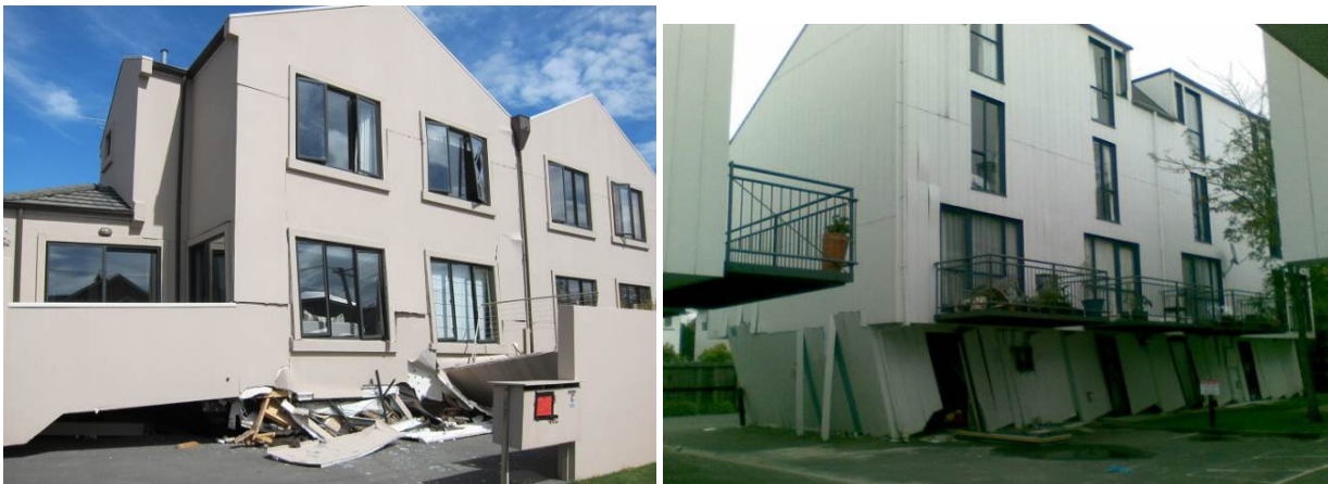
Figure 47: Timber buildings collapse/damage patterns: a) Soft-storey collapse of a relatively modern residential apartment; b) Soft-storey collapse of a four-storey residential apartment (Photo courtesy of Julian Ramsay)
