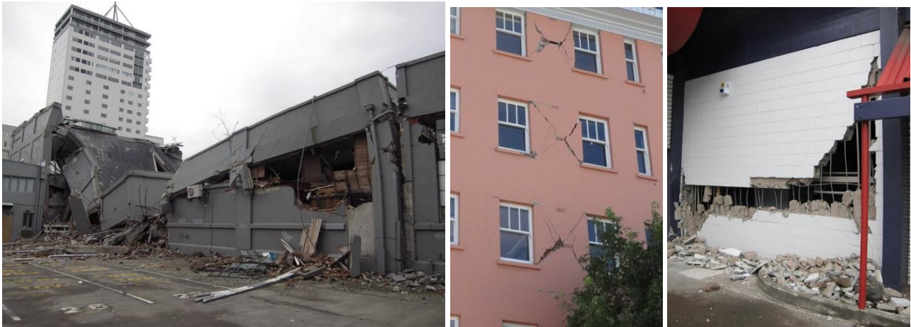
Figure 38: Reinforced concrete frame buildings collapse/damage patterns: a) 1930s three-storey RC frame with masonry infill collapsed after the 13 th June M w 6.2 aftershock; b) 1935 seven-storey RC frame with masonry infill and veneers; c) 1970s two-storey RC frame with reinforced concrete masonry blocks
