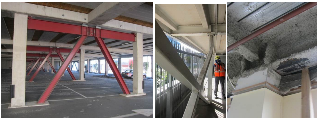
Figure 45: Steel frame and steel-braced buildings. collapse/damage patterns: a) Yielding and fracture of the shear-link of eccentric-braced frame with composite gravity frame; b) buckling and fracture of diagonal steel braces; c) Yield lines on steel-frame
