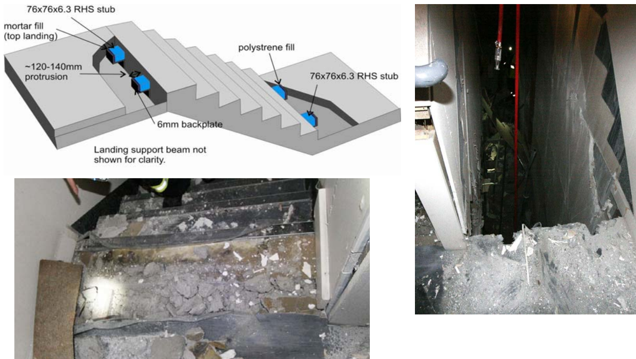
Figure 52: Alternative typical detailing of staircase- Type A - Pinned-slide connections with RHS shear keys on both ends and observed failures. (Damage photographs are courtesy of USAR teams)
