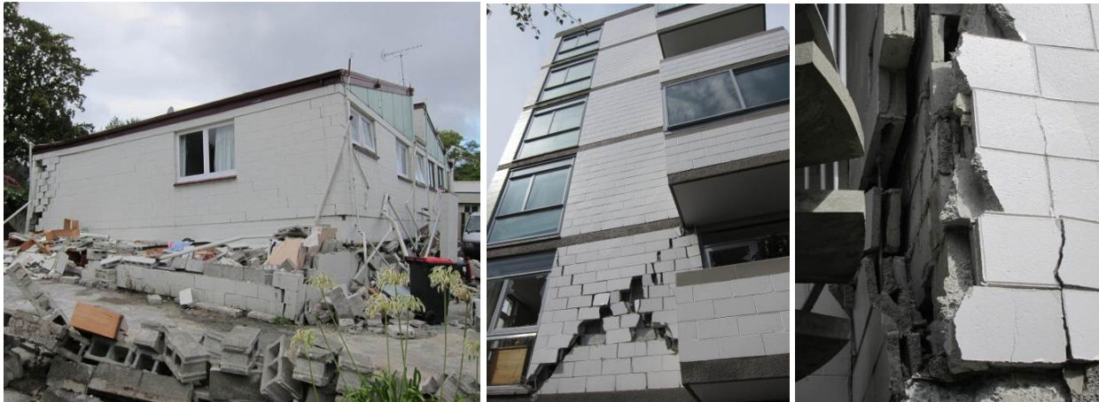
Figure 33: Reinforced concrete masonry buildings collapse/damage patterns: a) two-storey residential building with complete soft-storey collapse of the first floor; b-c) Shear failure of the 2 nd floor RCM walls of a six-storey residential apartment built in the 1960s
