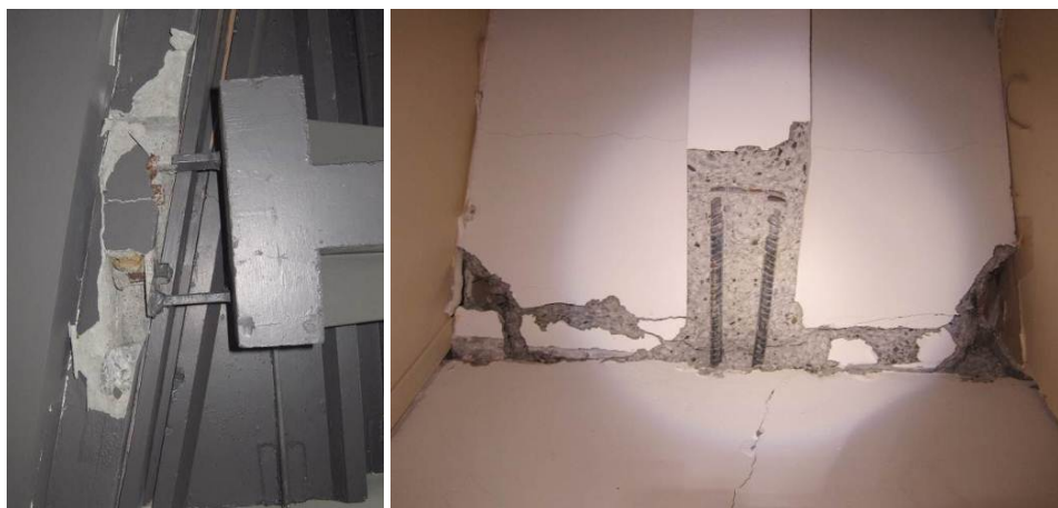
Figure 50: Bottom landing damage of precast concrete staircase in multi-storey buildings
