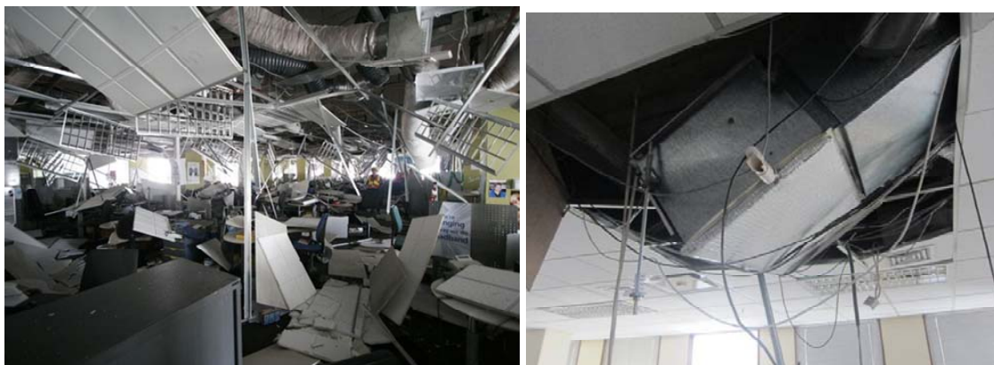
Figure 54: Damage and collapse of horizontal “non-structural elements”: a) Collapse of heavy ceiling tiles and services b) Near collapse of a HVAC unit due to anchorage failure
