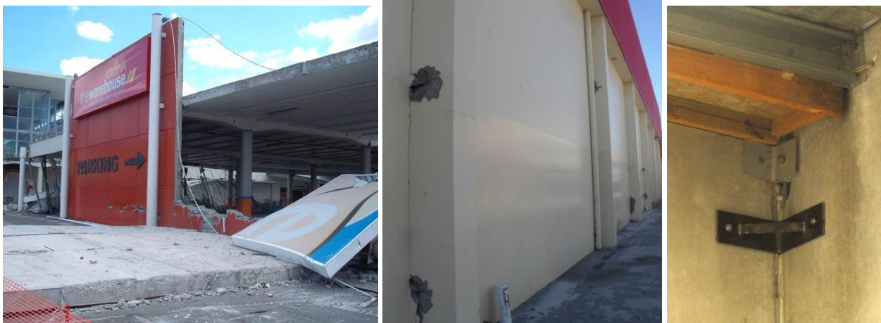
Figure 43: Tilt-up concrete wall buildings collapse/damage patterns: a) Failure of the spliced-connection of the tilt-up panel walls (photo courtesy of John Marshall); b) Tilt-up panels with encased steel portal frame; c) Steel angle connection damaged in the 4 th Sept earthquake, repaired with a supplementary bolted steel angle
