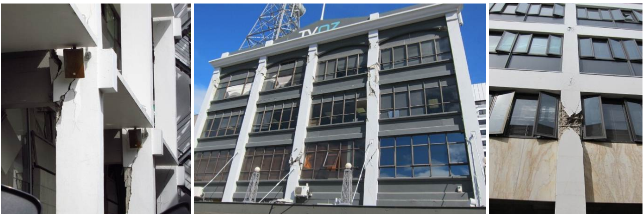
Figure 35: Pre-1970s reinforced concrete moment-resisting frame buildings collapse/damage patterns
