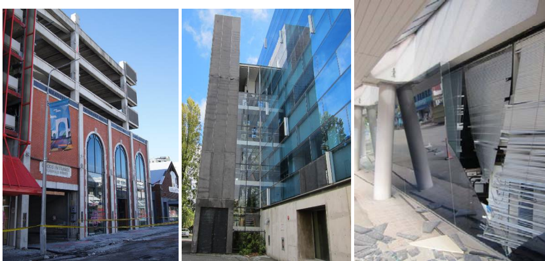
Figure 53: Damage and collapse of vertical “non-structural elements”: a) Collapse of heavy precast concrete panels due to failure of the connecting bolted-plates; b) The failure of the inter-panel shear connection of an external lift-shaft located next to the only safety egress for the building; c) Shattered glass façade at street retail level
