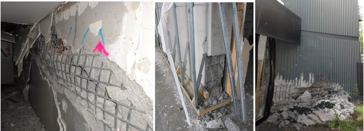
Figure 41: Post-1970s reinforced concrete structural wall buildings collapse/damage patterns: a) Nine-storey residential apartment built in 2000-2010 with severe shear failure of the long slender wall (photo courtesy of Ken Elwood); b) 14-storey residential apartment built in 2007 with buckling of the boundary reinforcements; c) Seven-storey 1980s office block with significant compression failure of the V-shaped RC shear wall
