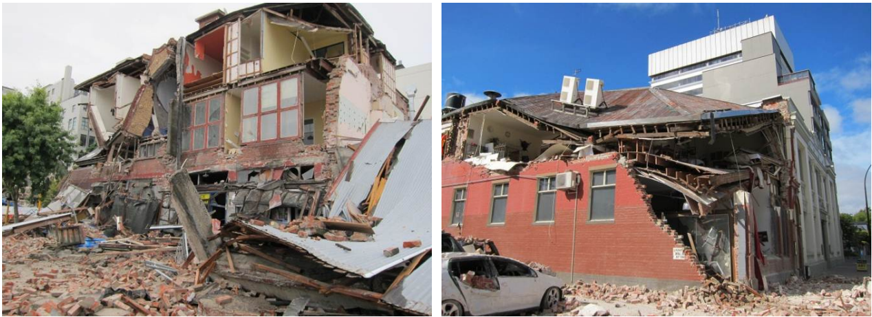
Figure 29: Unreinforced masonry buildings collapse/damage patterns: Mixed of in-plane and out-of-plane failure modes
