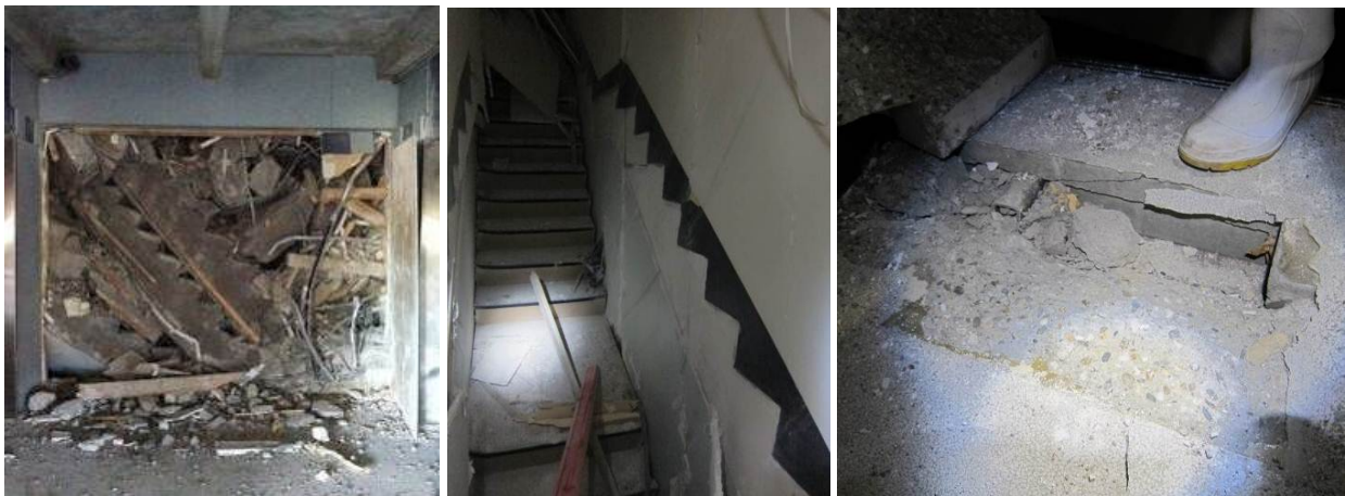
Figure 49: Collapse (a-b) and top landing damage (c) of precast concrete staircase in multi-storey buildings
