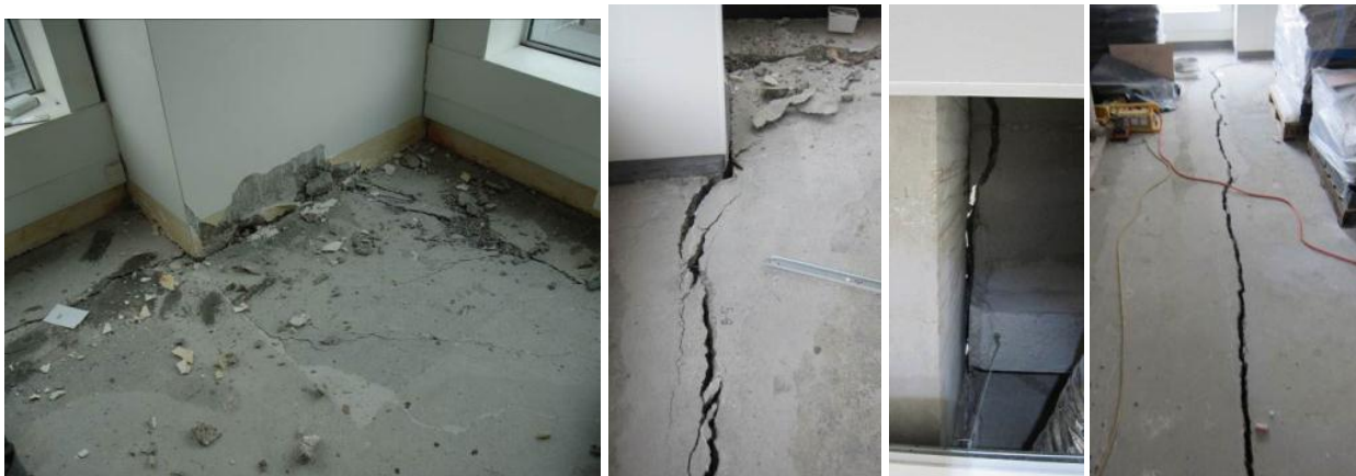
Figure 55: Extensive damage of floor diaphragm and loss of floor support due to the beam-elongation effects of concrete frame inelastic response
