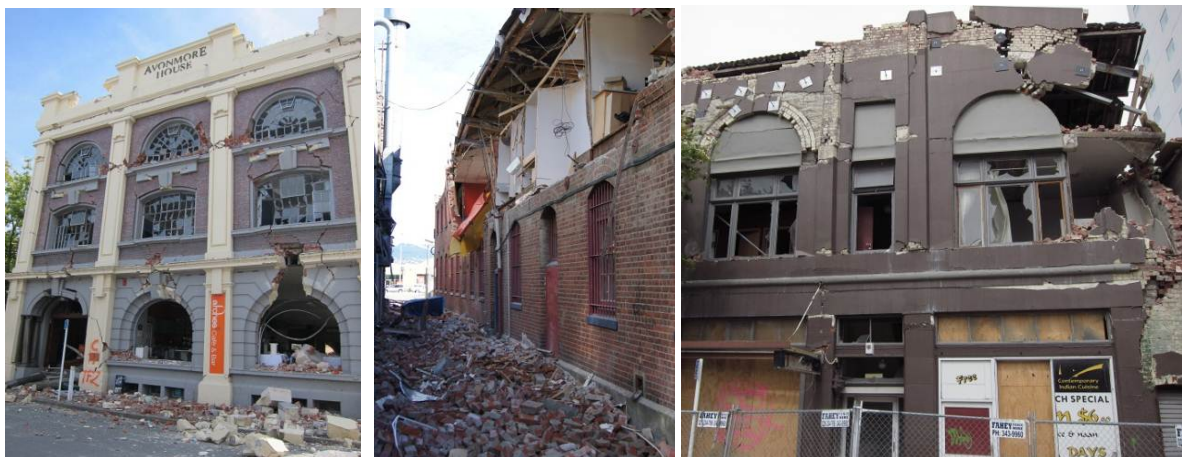
Figure 30: Unreinforced masonry buildings collapse/damage patterns: Mixed of in-plane and out-of-plane failure modes
