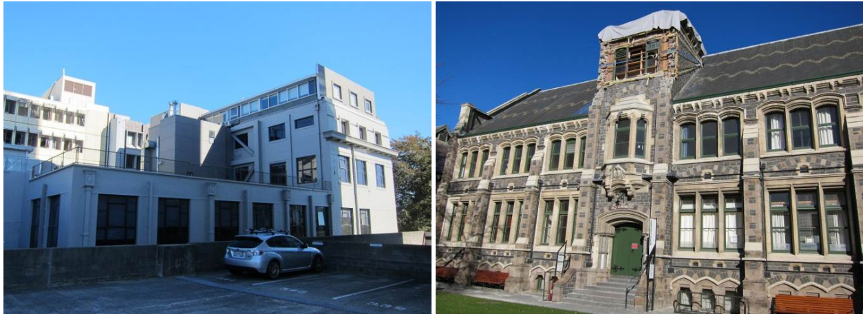
Figure 31: Good performance of seismic retrofitted unreinforced masonry and brick buildings: a) Public Trust Building; additional external steel braces and internal RC walls; b) Art Centre’s Old Chemistry Building; external horizontal and vertical post-tensioning, with closely spaced tie-in rose anchors
